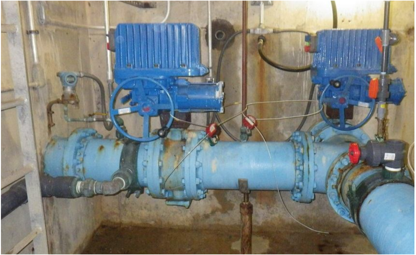
9. Piping and valves in vault.
