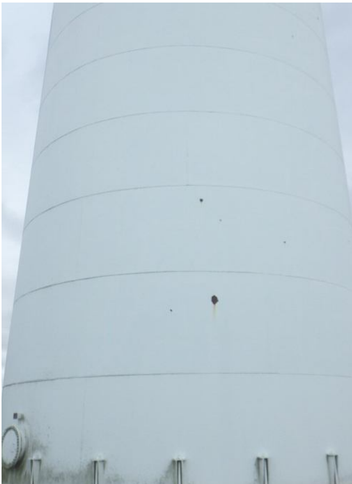
24. Coating failures and rust on shell.
