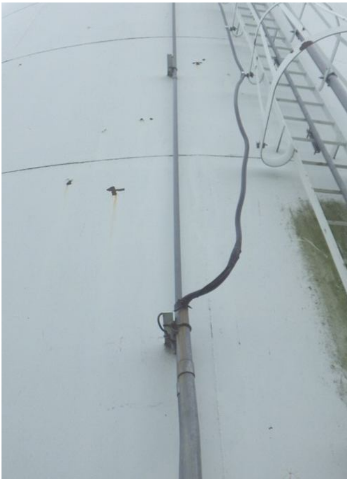
29. Conduit and coaxial cable adjacent to shell ladder.
