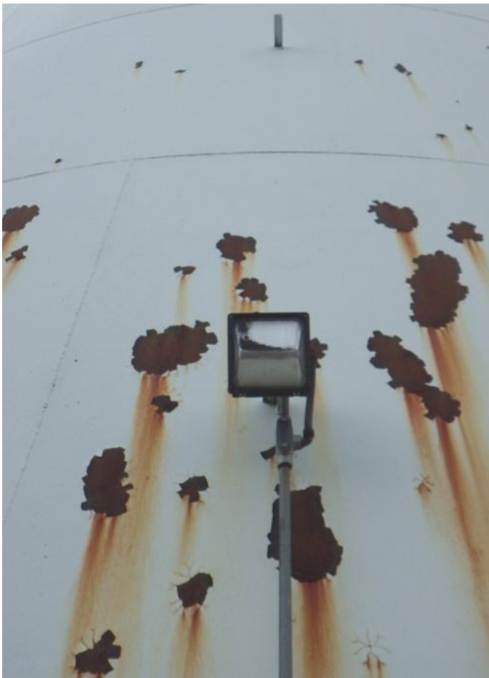
23. Light fixture. Note coating failures and rust on shell.
