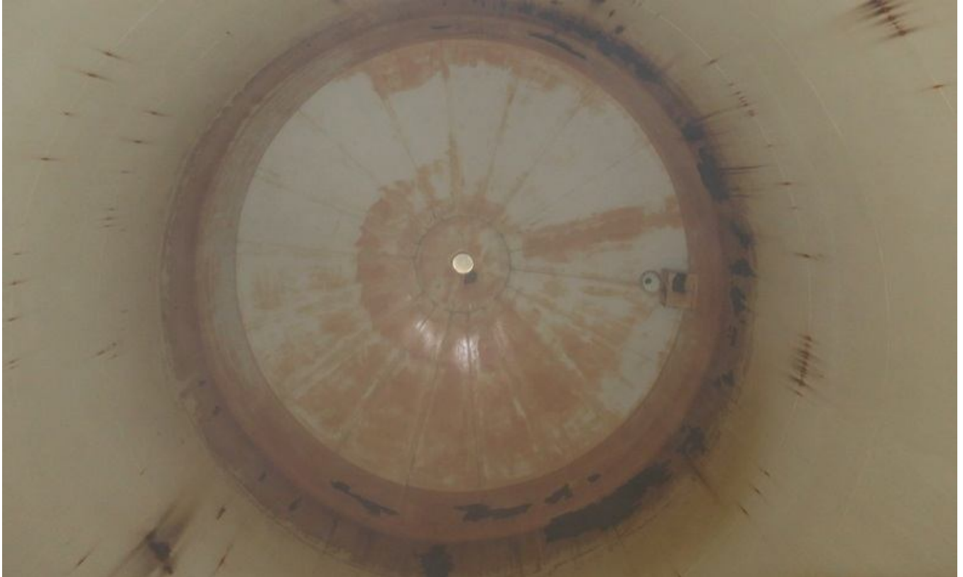
48. Interior roof and shell. Note corrosion.
