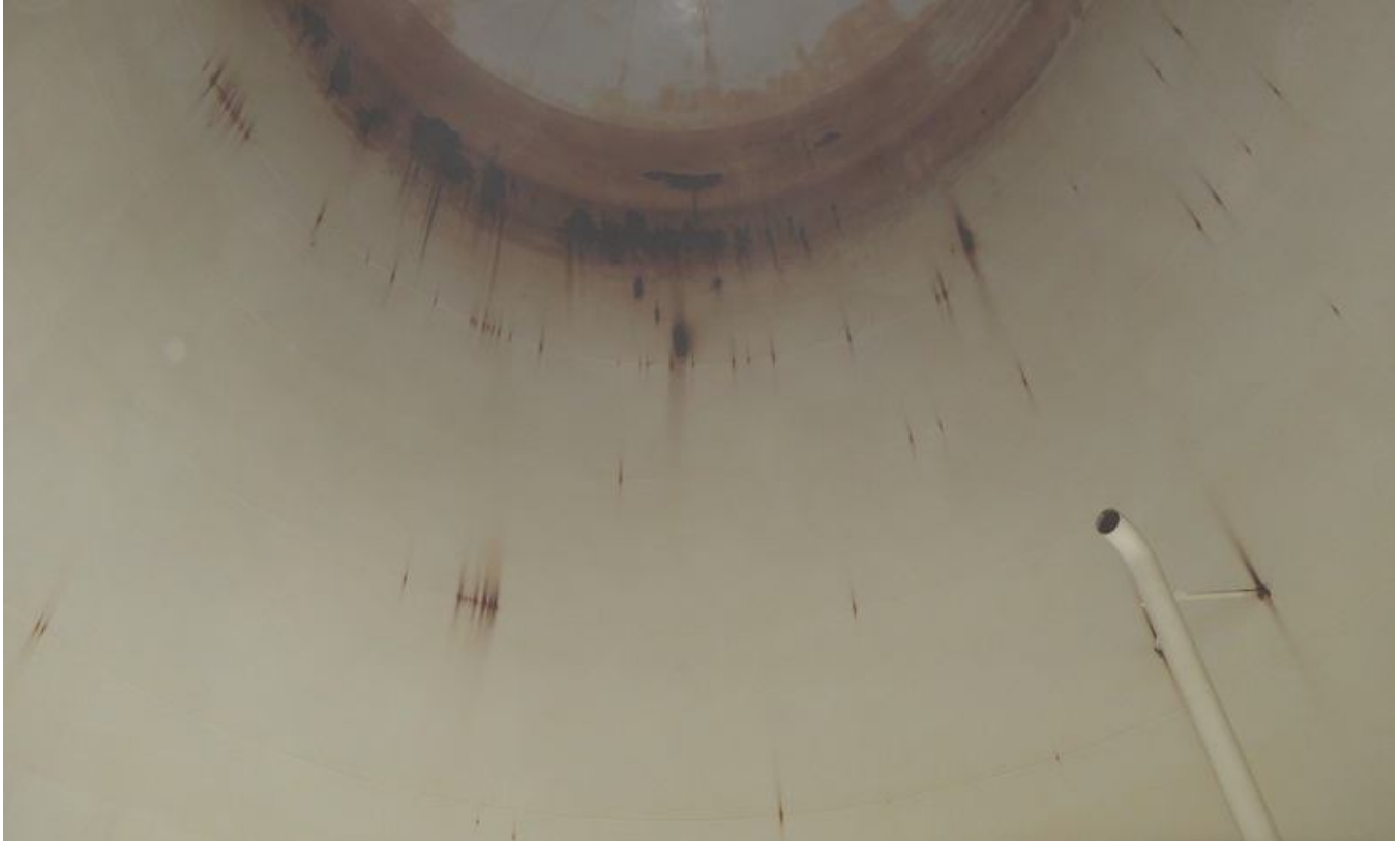
56. Corrosion on interior shell.
