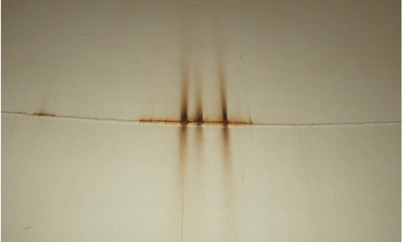
54. Corrosion along interior shell weld seam.
