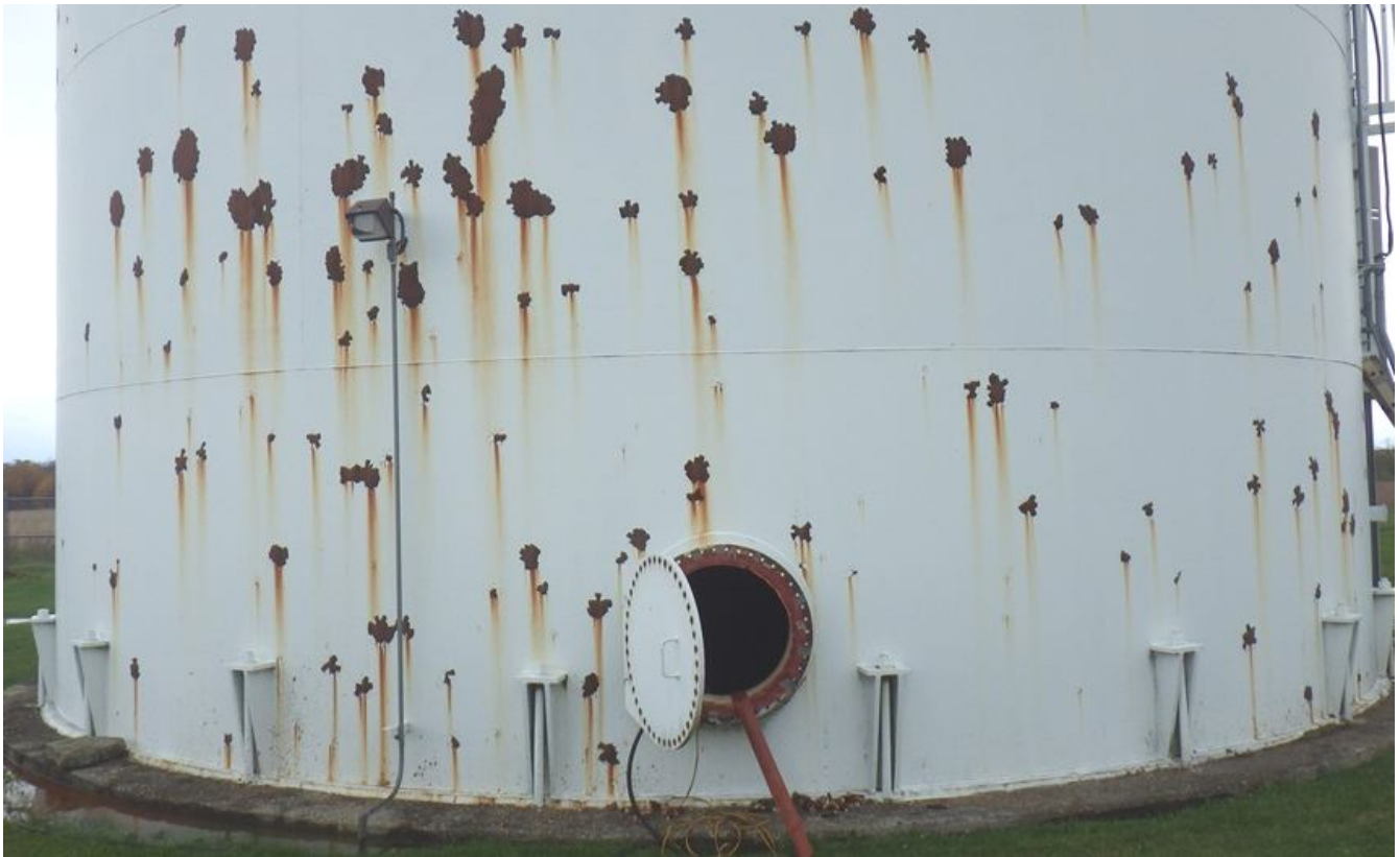
22. Shell manhole and light fixture. Note coating failures and rust on shell.
