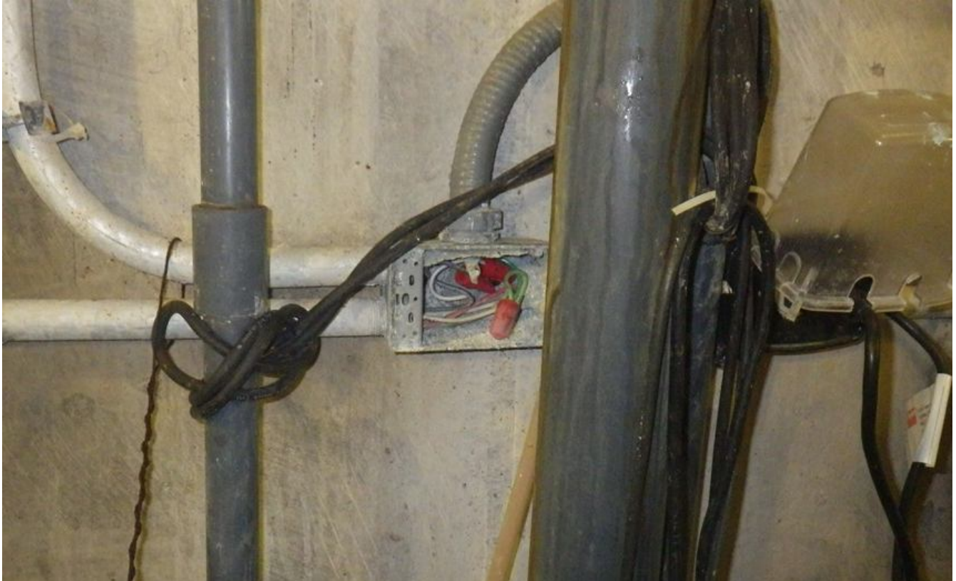
10. Conduit junction with missing cover.
