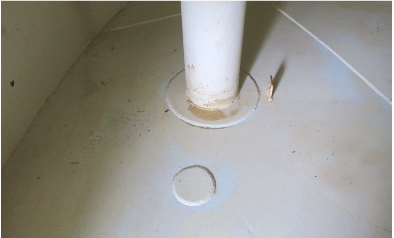
63. Inlet pipe at floor.
