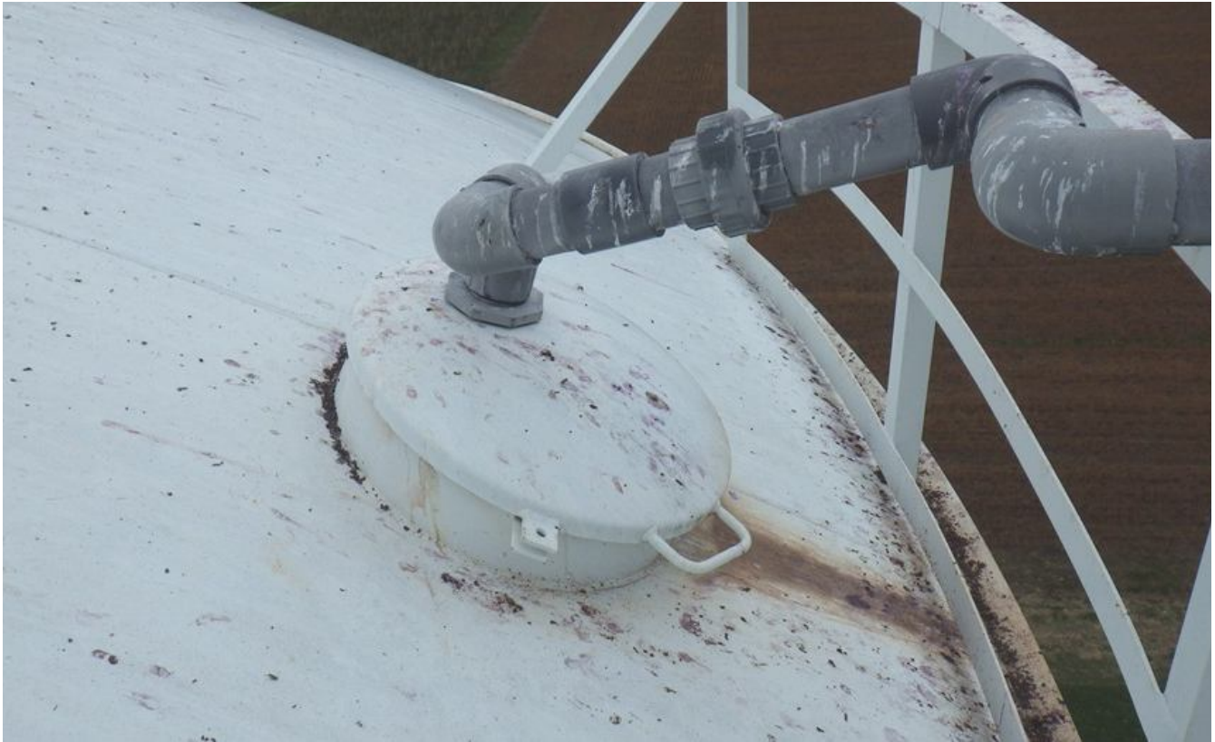
35. Pipe attached to hinged roof manhole cover.
