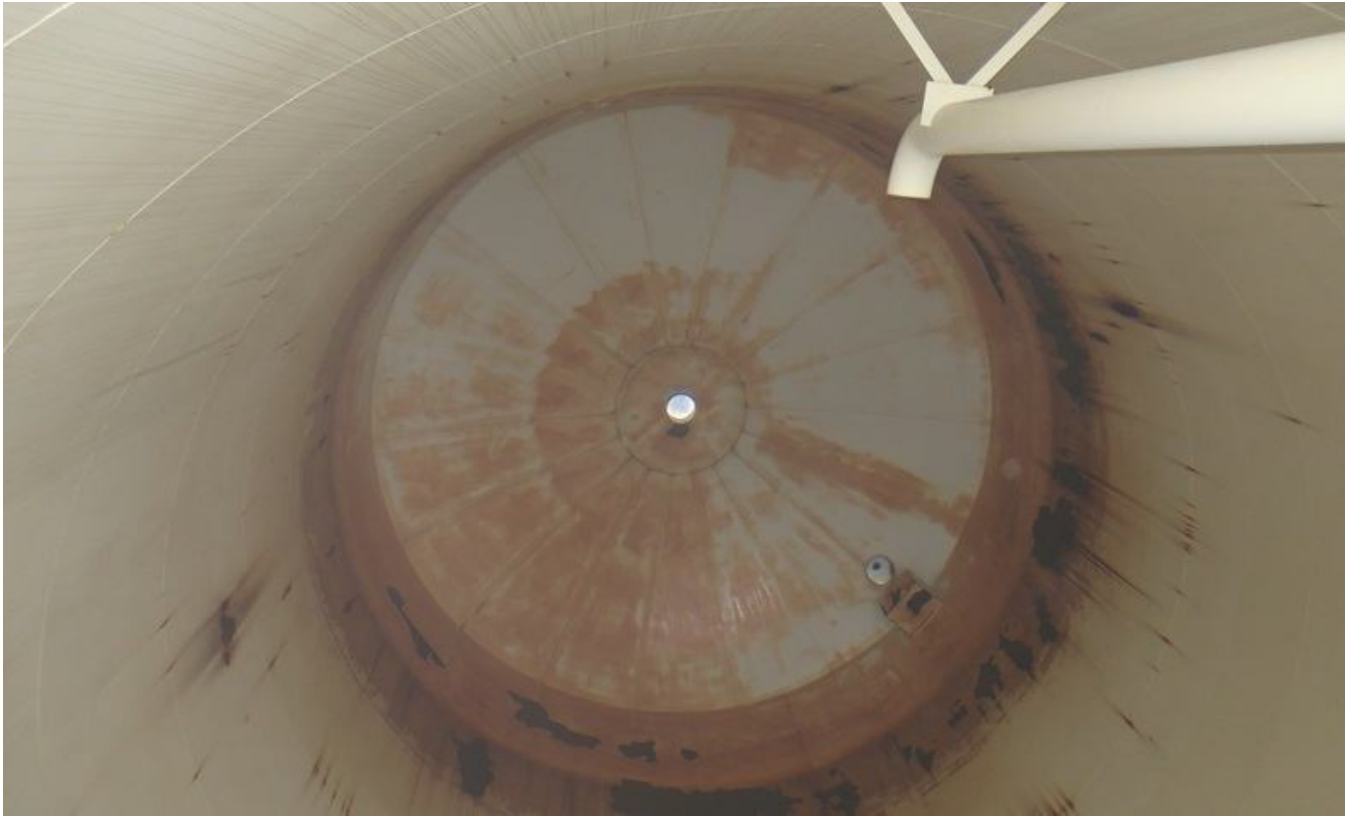
49. Interior roof, shell, and inlet pipe. Note corrosion.
