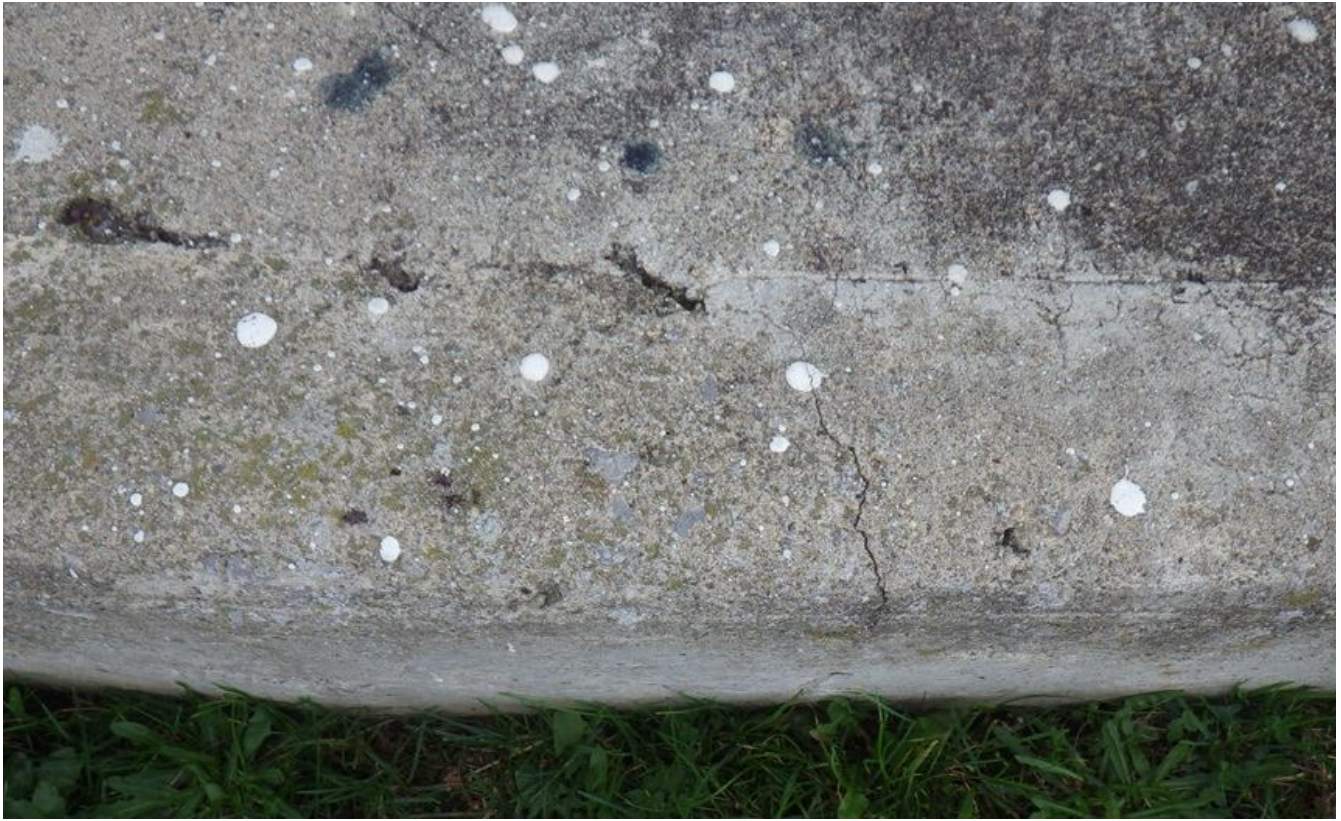
11. Crack in tank foundation.
