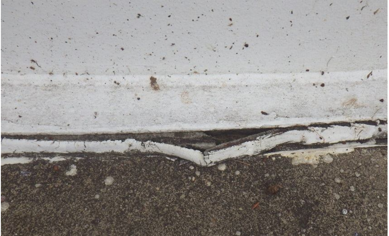
14. Peeled sealant along grout and bottom plate.
