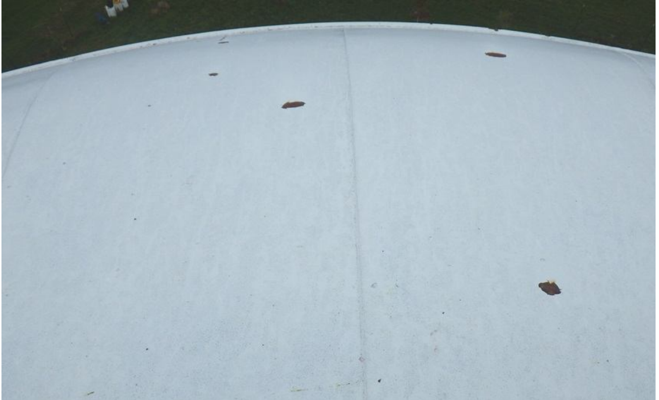
38. Coating failures and rust on exterior roof.
