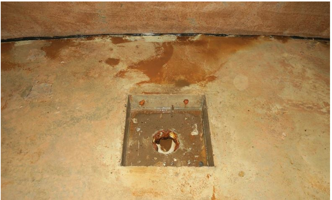
58. Corrosion on piping in sump.
