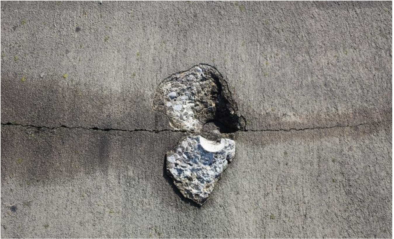
33. Spalling and cracking in roof.
