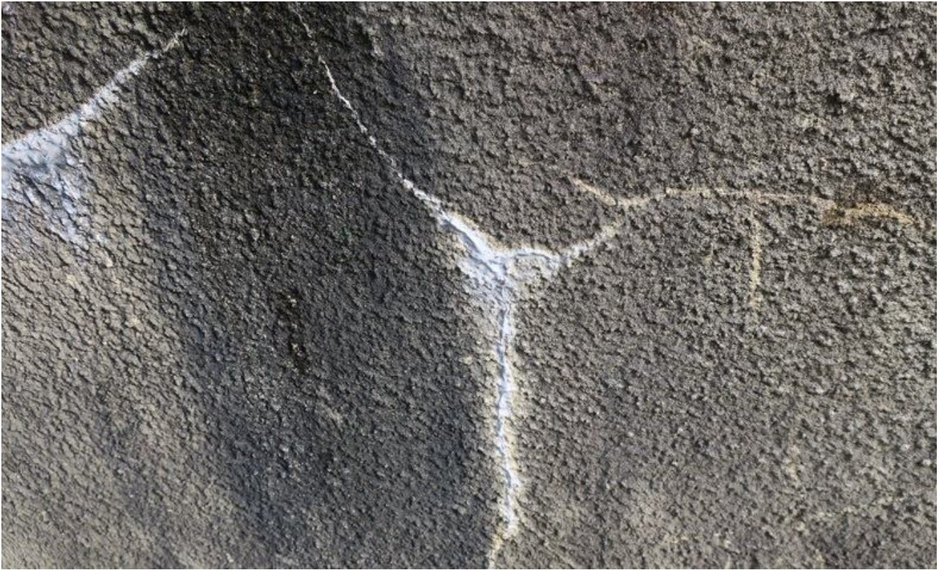
15. Efflorescence on shell.
