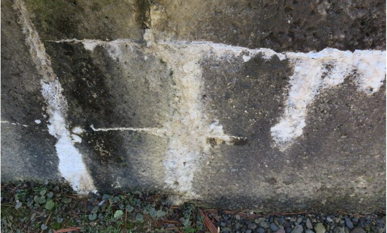
16. Efflorescence on shell.
