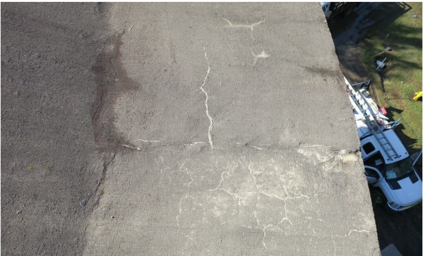
28. Efflorescence in roof.
