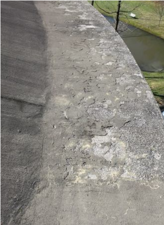
27. Surface deterioration in roof perimeter.
