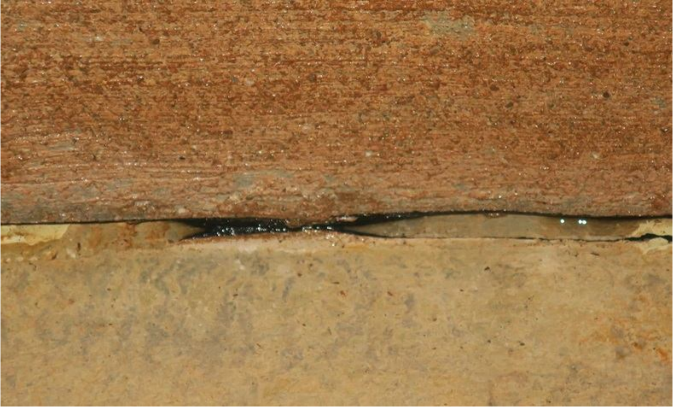
54. Voids in material along shell-to-floor connection.
