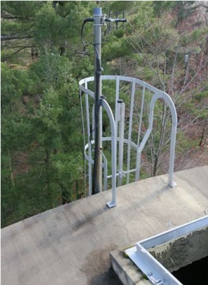
25. Antenna and roof access.
