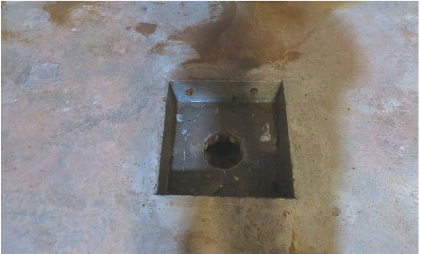
59. Piping in sump.
