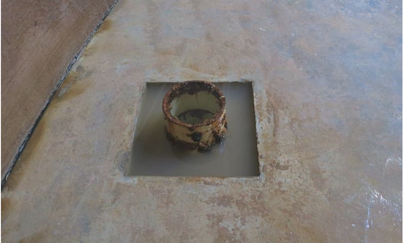
60. Corrosion on piping in sump.
