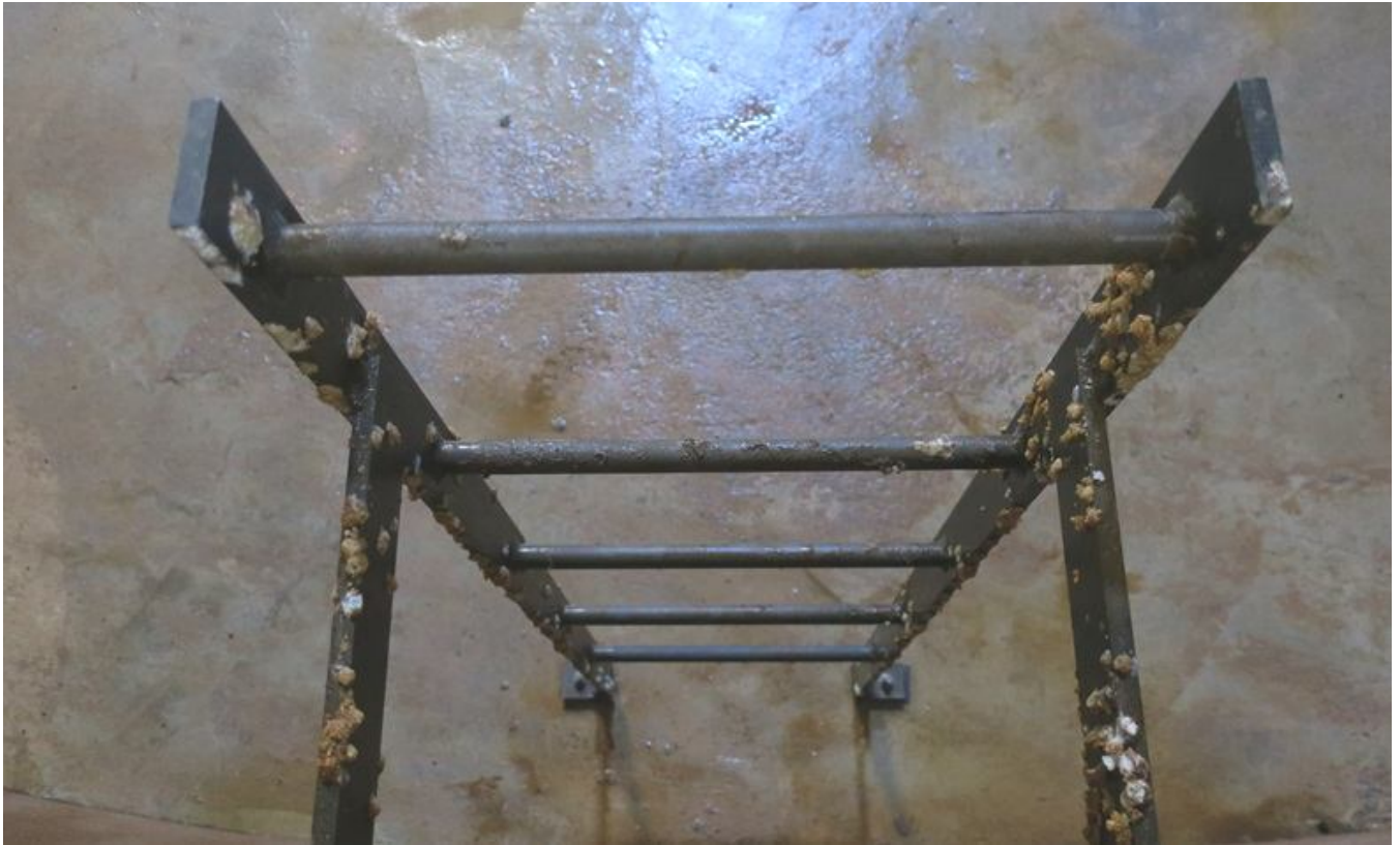
53. Deposits on interior ladder.
