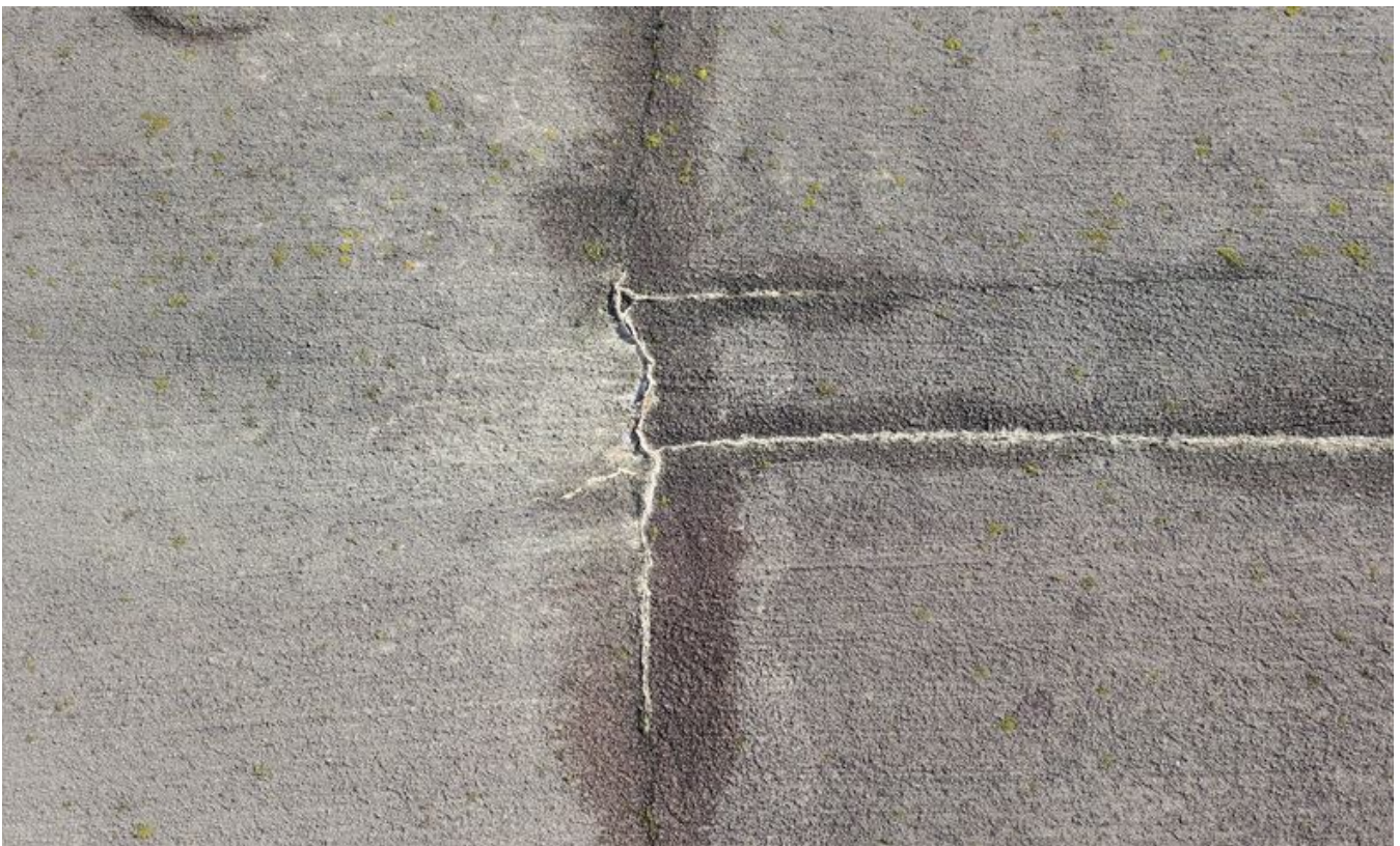
32. Efflorescence on roof.
