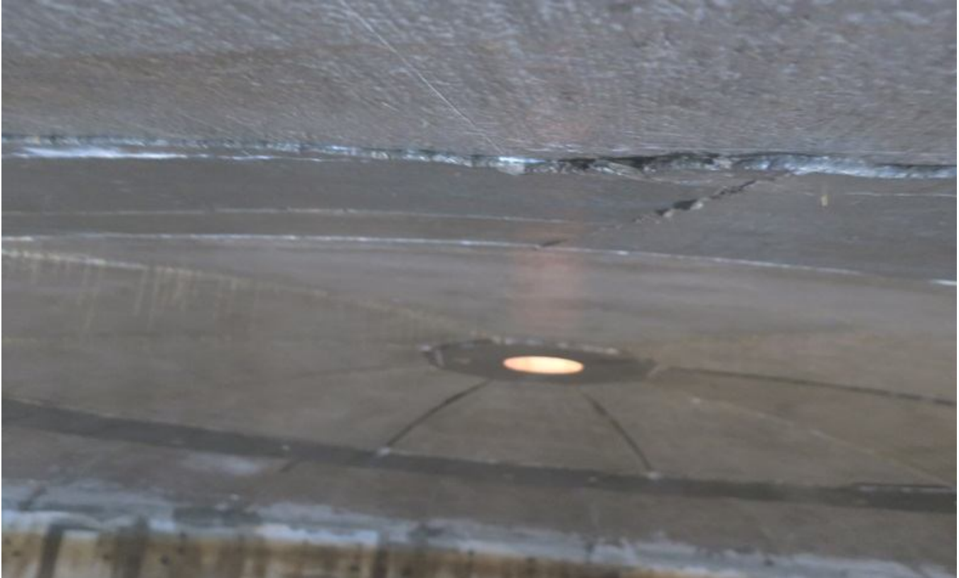
38. Crack in roof.
