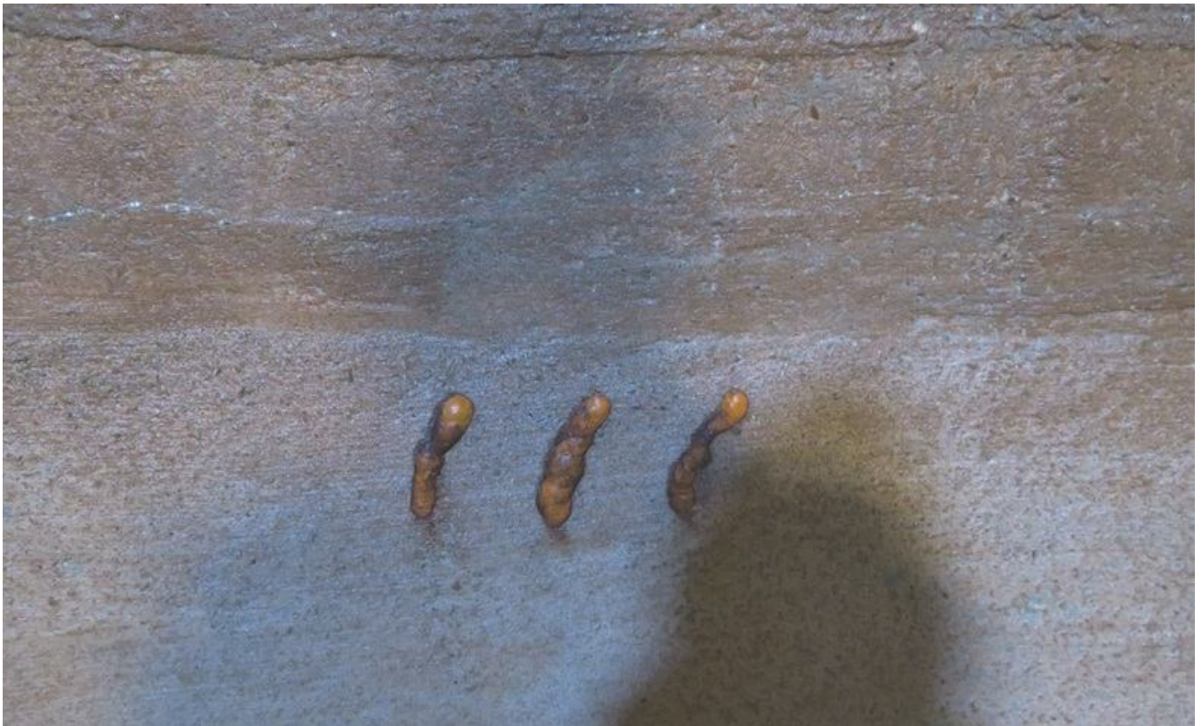
48. Rust tubercles at exposed steel in shell.
