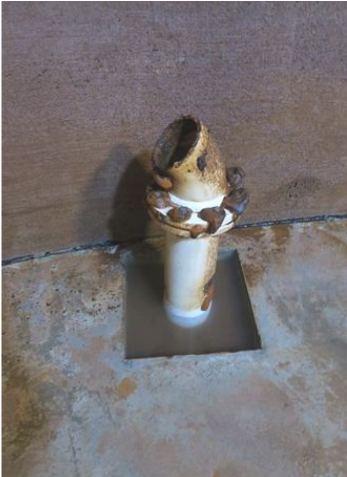
57. Corrosion on interior pipe projection.
