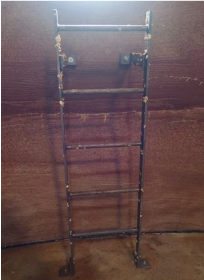
51. Deposits on interior ladder.
