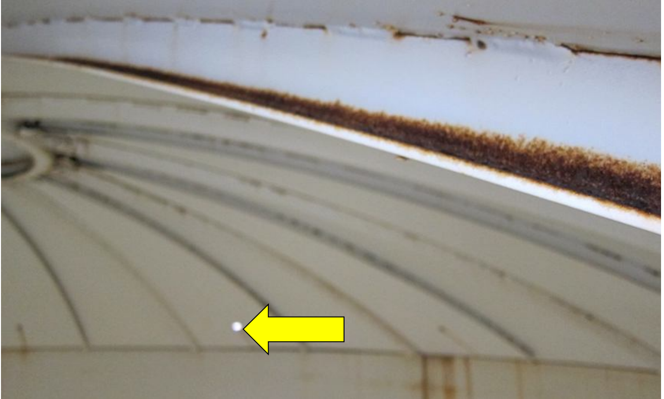
40. Corrosion along roof stiffener. Note daylight at coupling opening.
