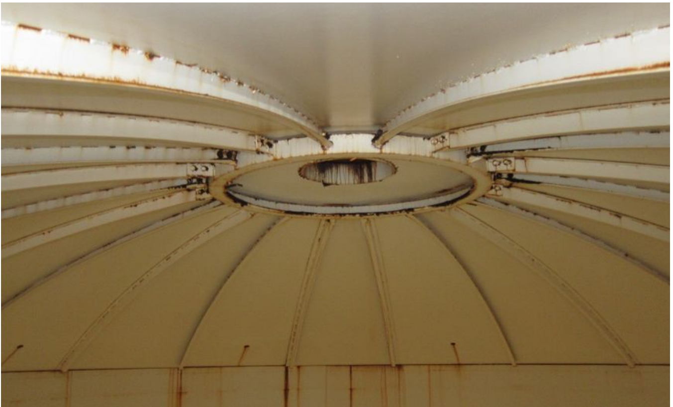
38. Corrosion on roof stiffeners.
