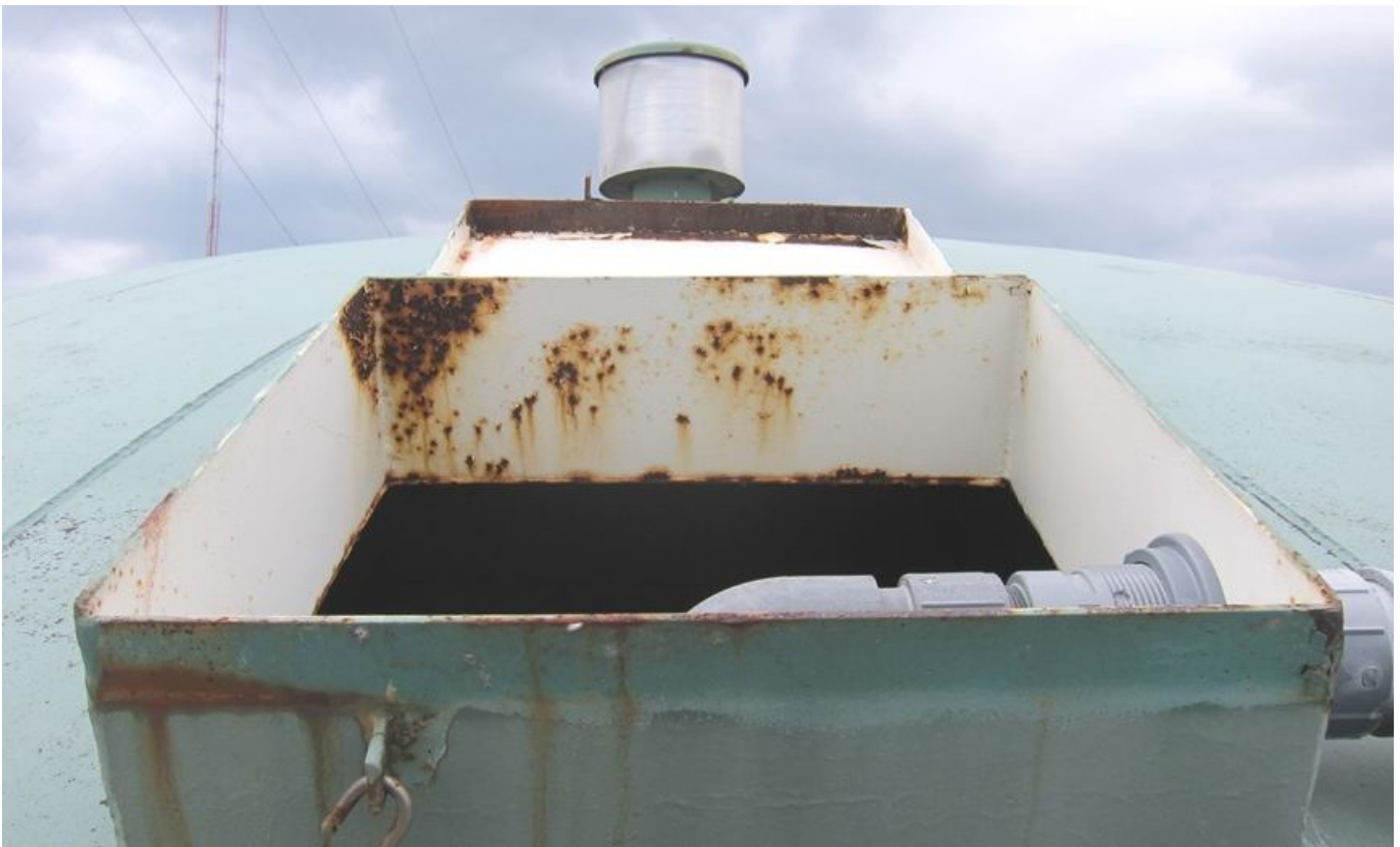
28. Corrosion on roof manhole.
