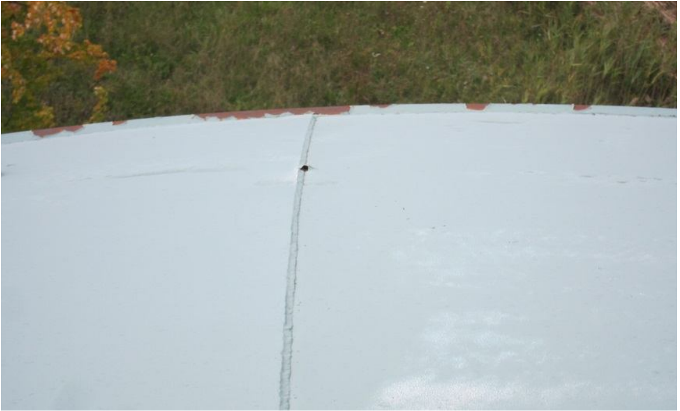
31. Peeled coating and corrosion along roof perimeter.
