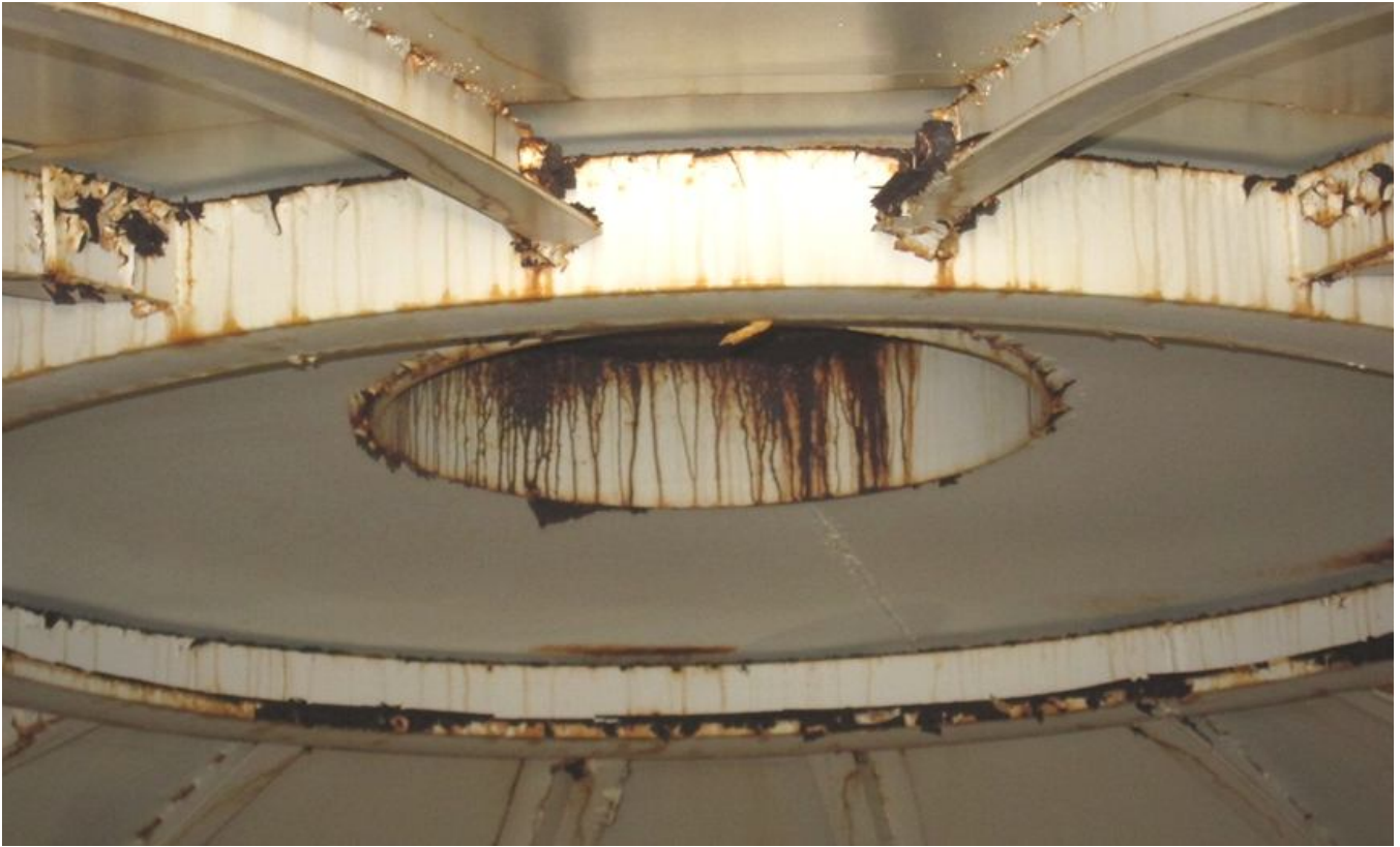
39. Corrosion and metal loss along roof stiffeners and around roof vent opening.
