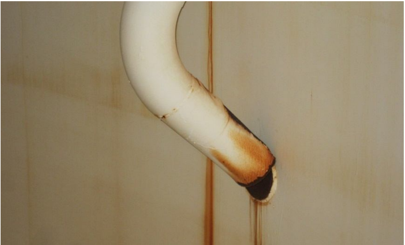
44. Overflow pipe no longer attached to shell.
