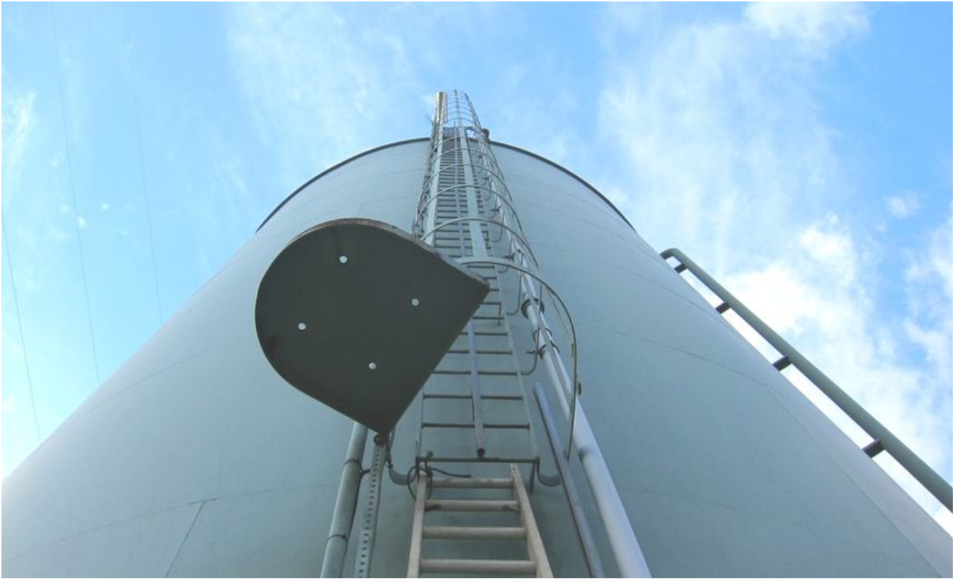
19. Vandal deterrent at base of exterior ladder.
