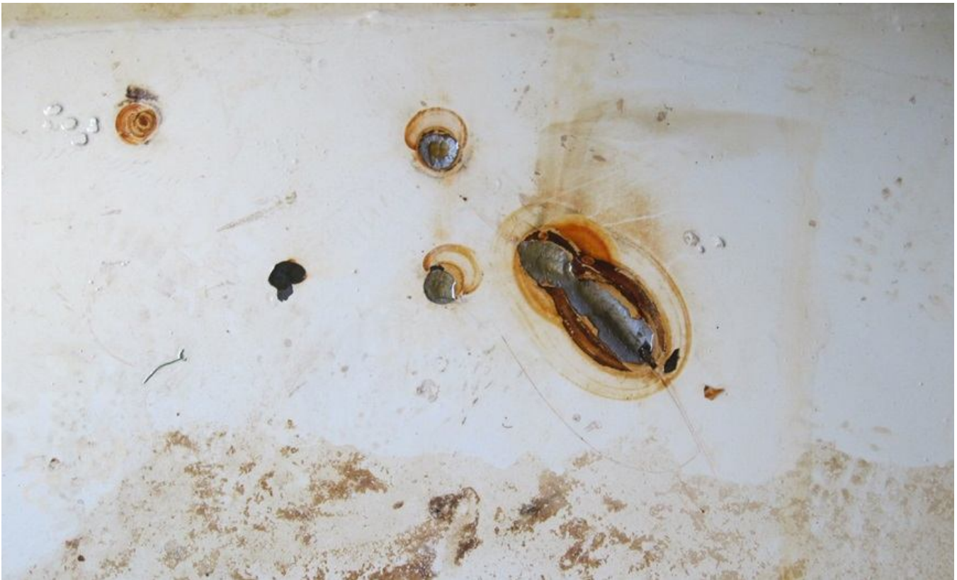
52. Metal loss in floor.
