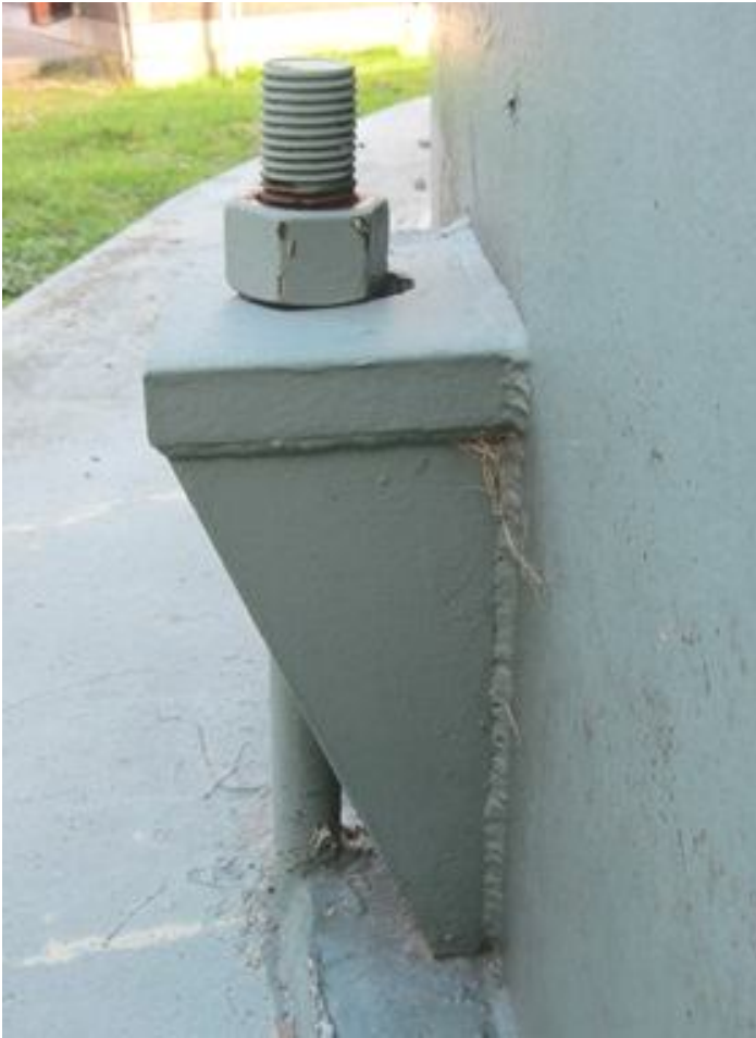
11. Anchor bolt and chair. Note gap at nut-to-top plate interface.
