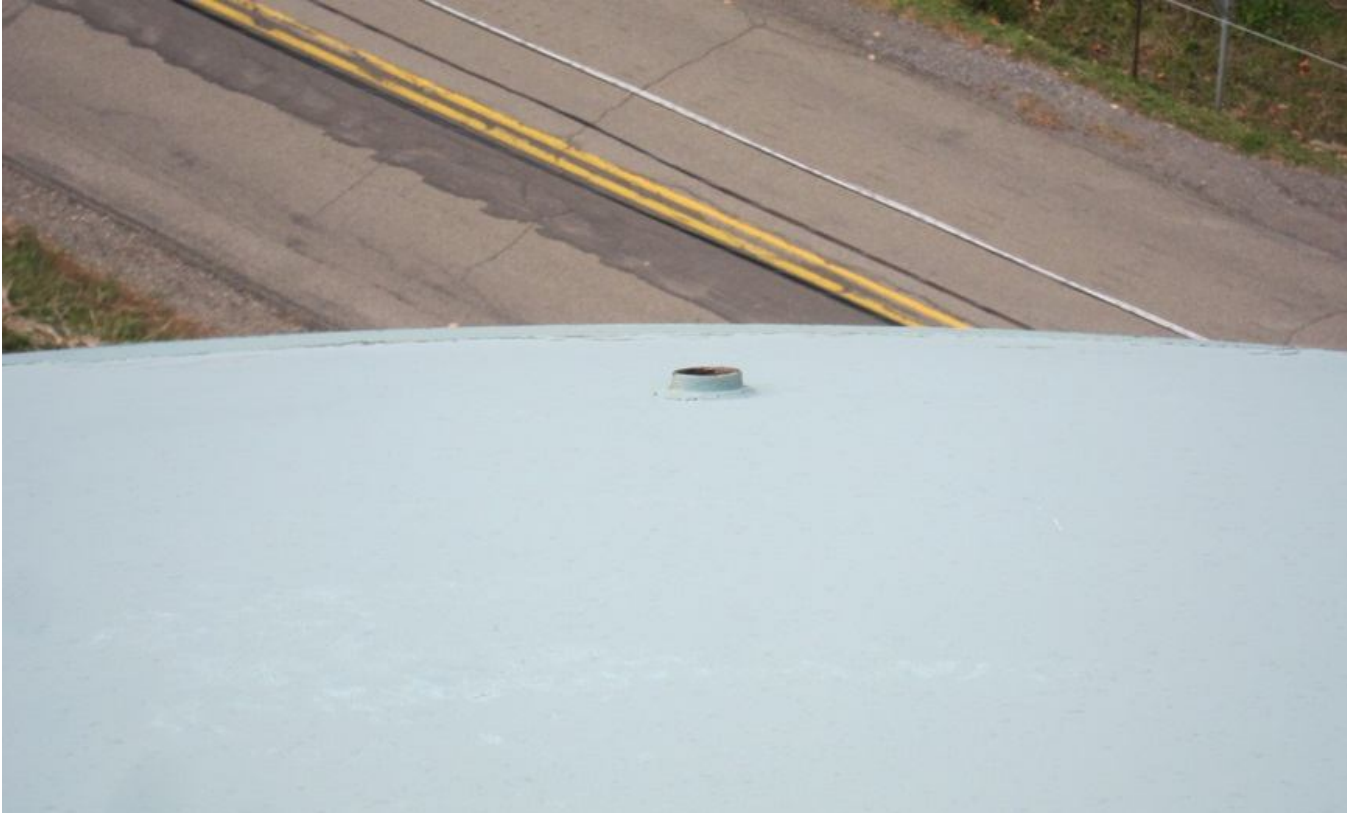
32. Open roof coupling.
