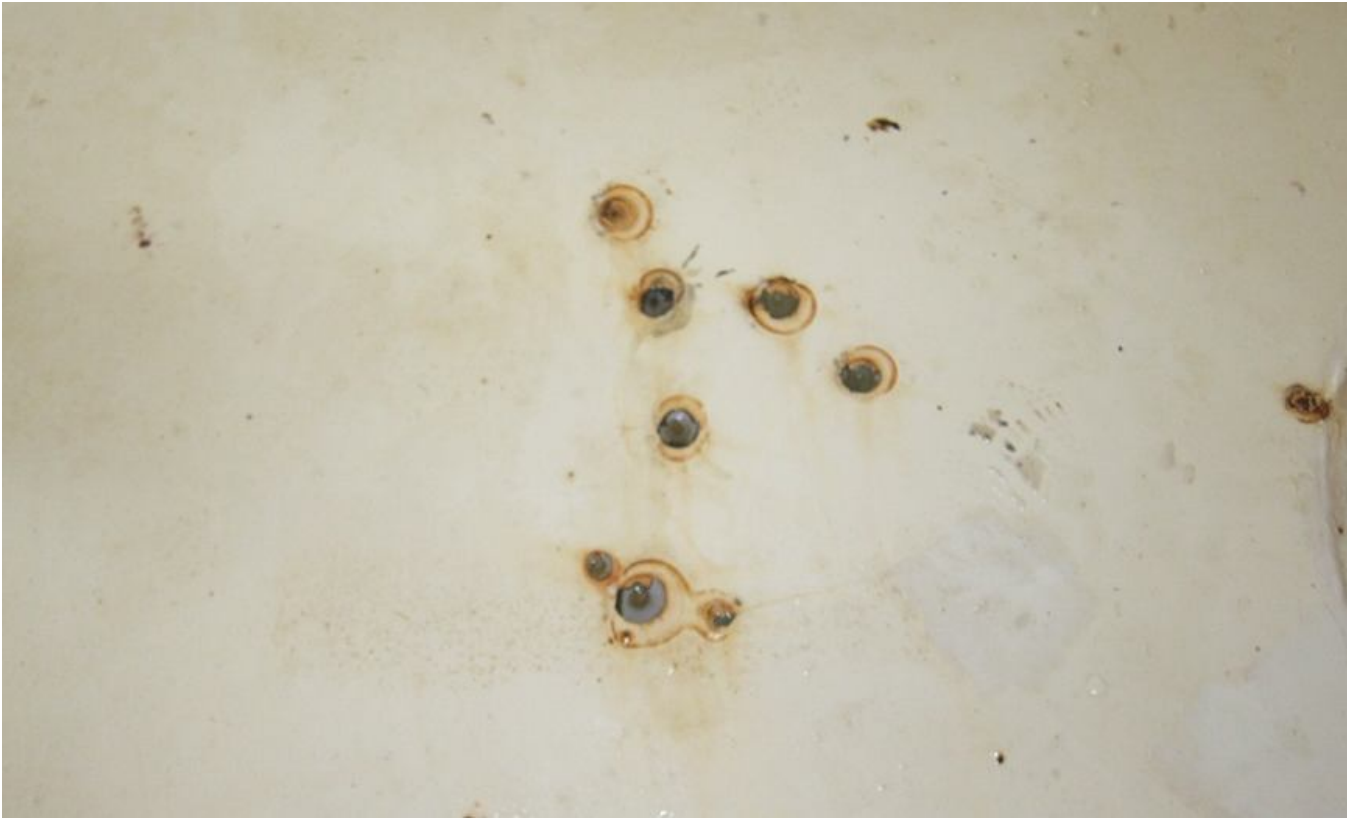
51. Metal loss in floor.
