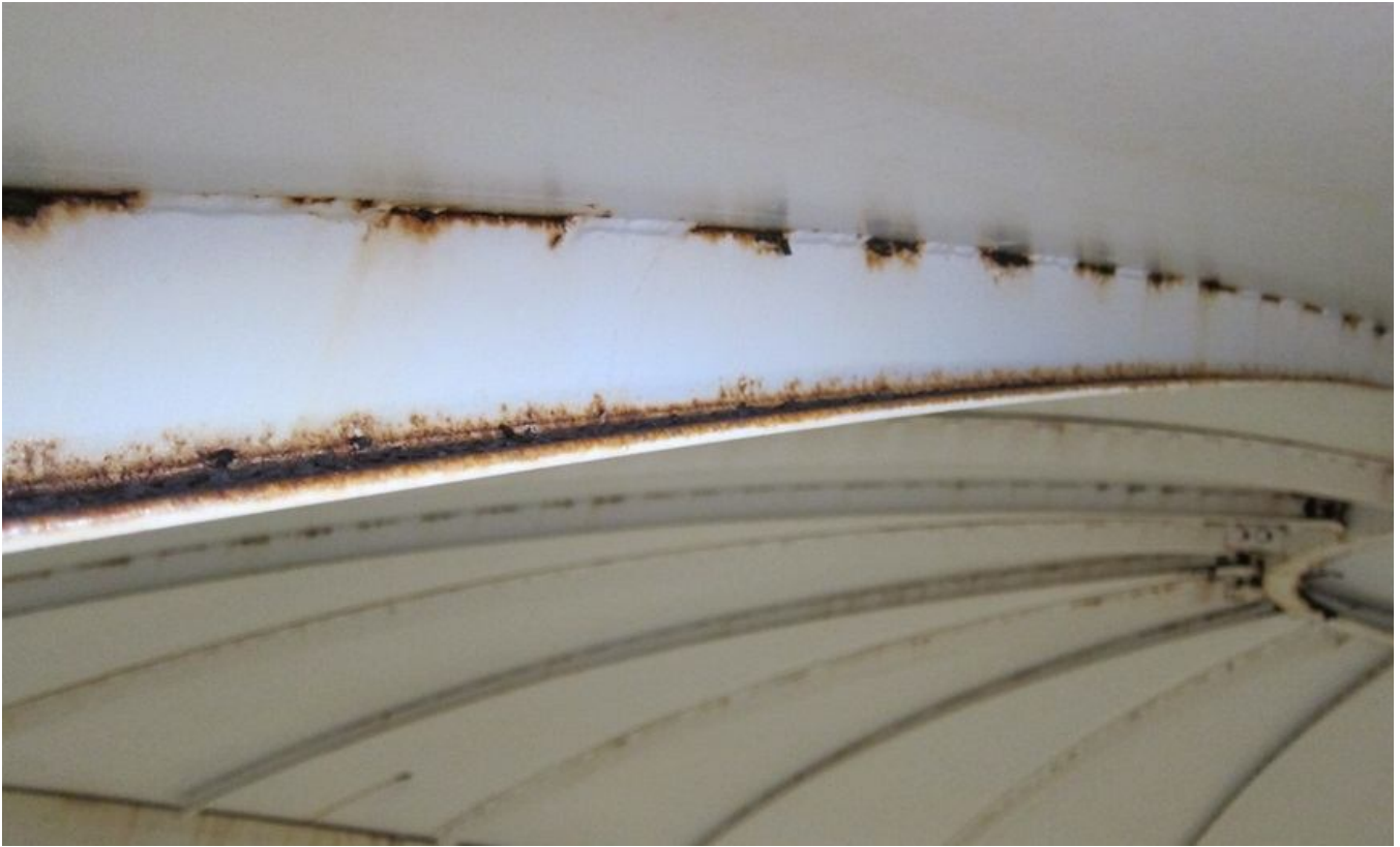
41. Corrosion along roof stiffener.
