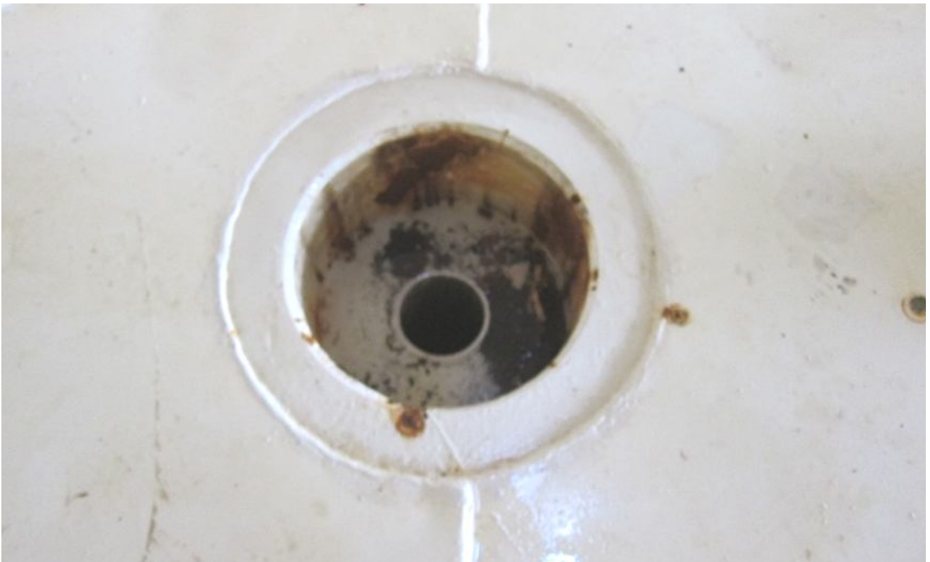
56. Drain pipe in sump.
