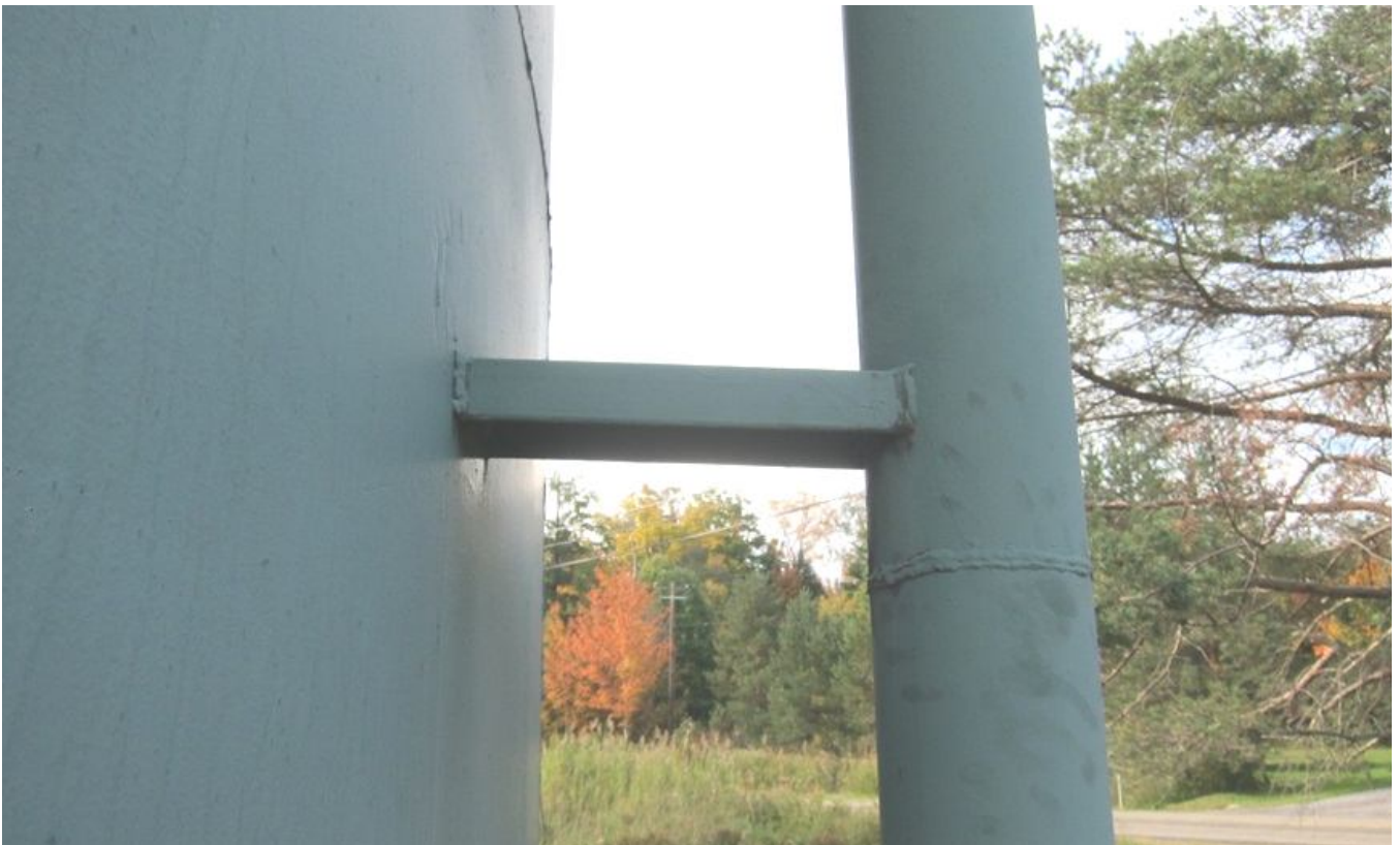
18. Overflow pipe and bracket.
