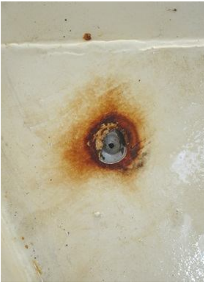
53. Hole in floor.
