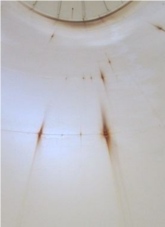
47. Corrosion along shell horizontal seams.
