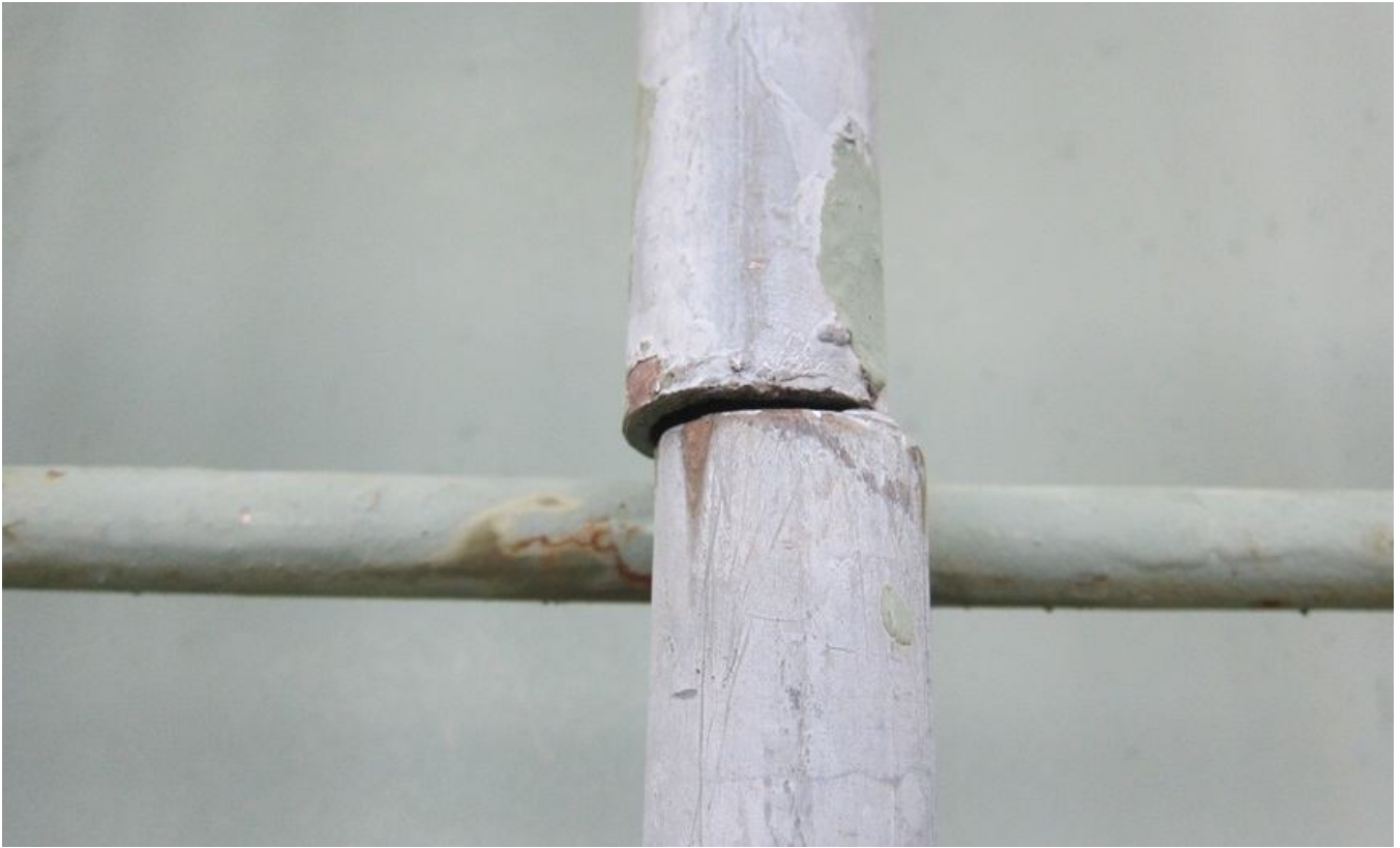
23. Misaligned notched-tubular rail sections.
