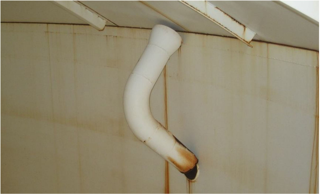
43. Overflow pipe no longer attached to shell.
