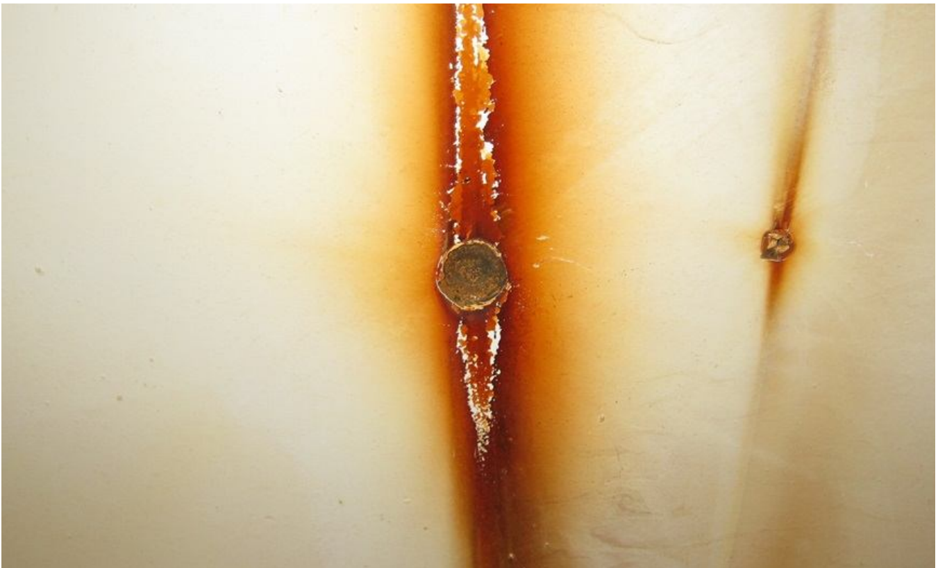
48. Corrosion and metal loss in shell.
