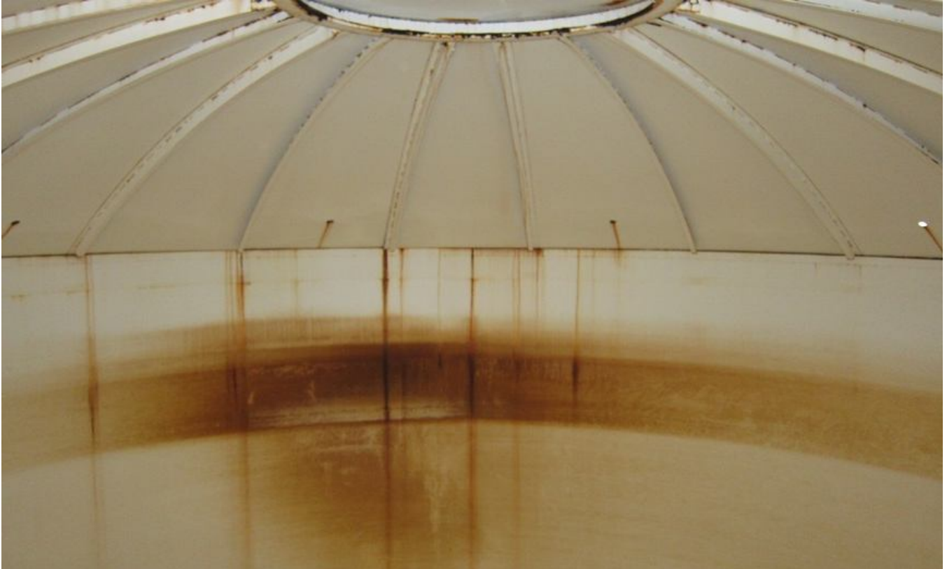
42. Roof and rust staining on upper shell.
