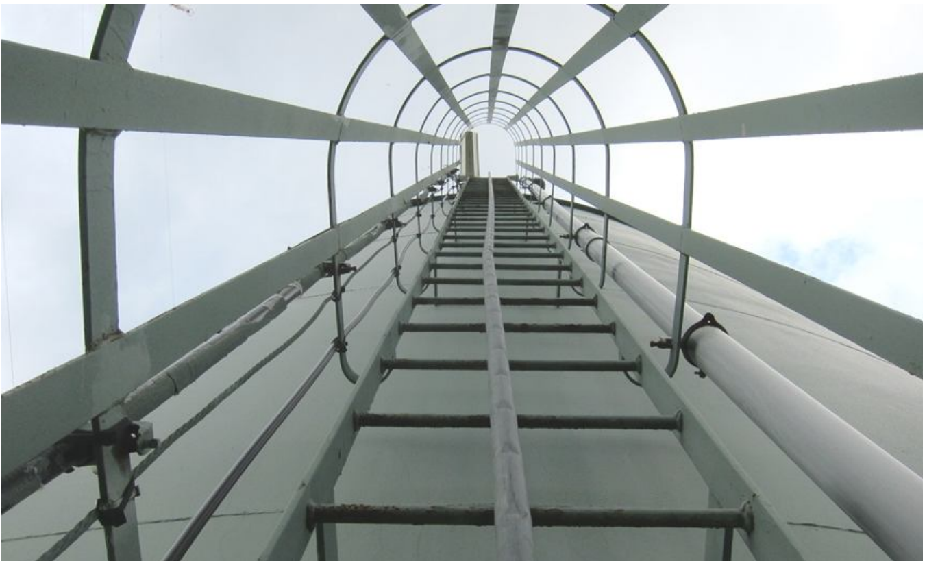
20. Exterior ladder, conduit, cables, safe-climbing device, PVC, and safety cage.
