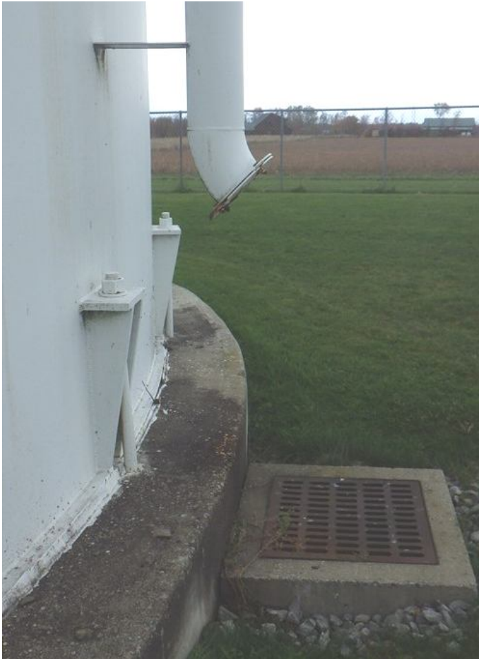
25. Overflow pipe discharge above drain basin.
