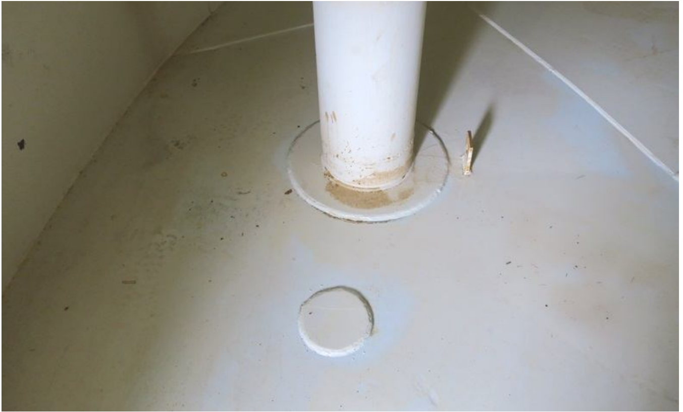
63. Inlet pipe at floor.
