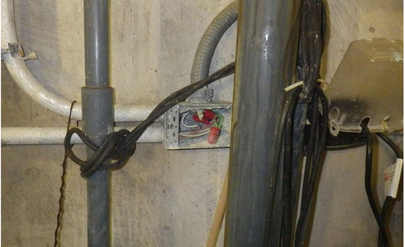
10. Conduit junction with missing cover.
