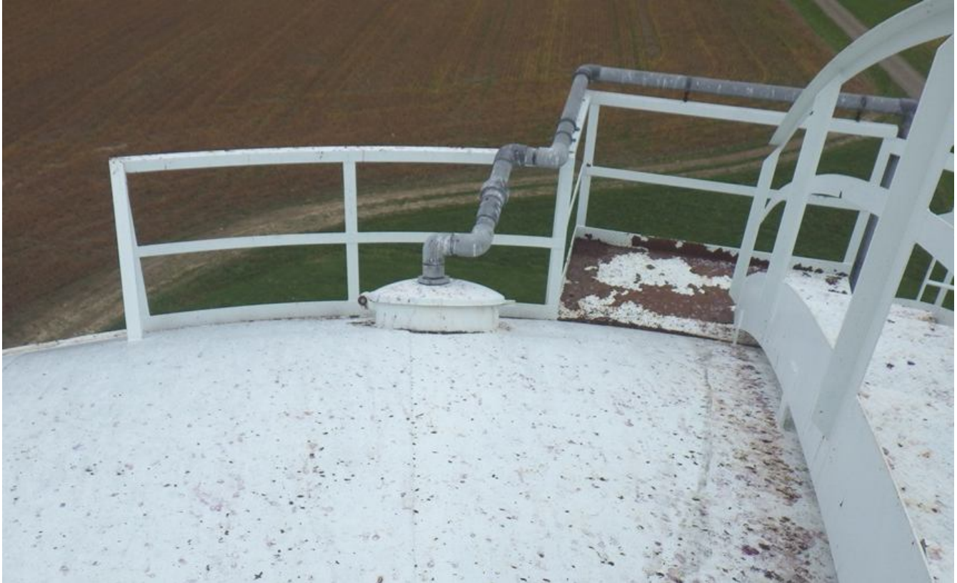
36. Roof safety railing, platform, stairs, and pipe attached to hinged roof manhole cover.
