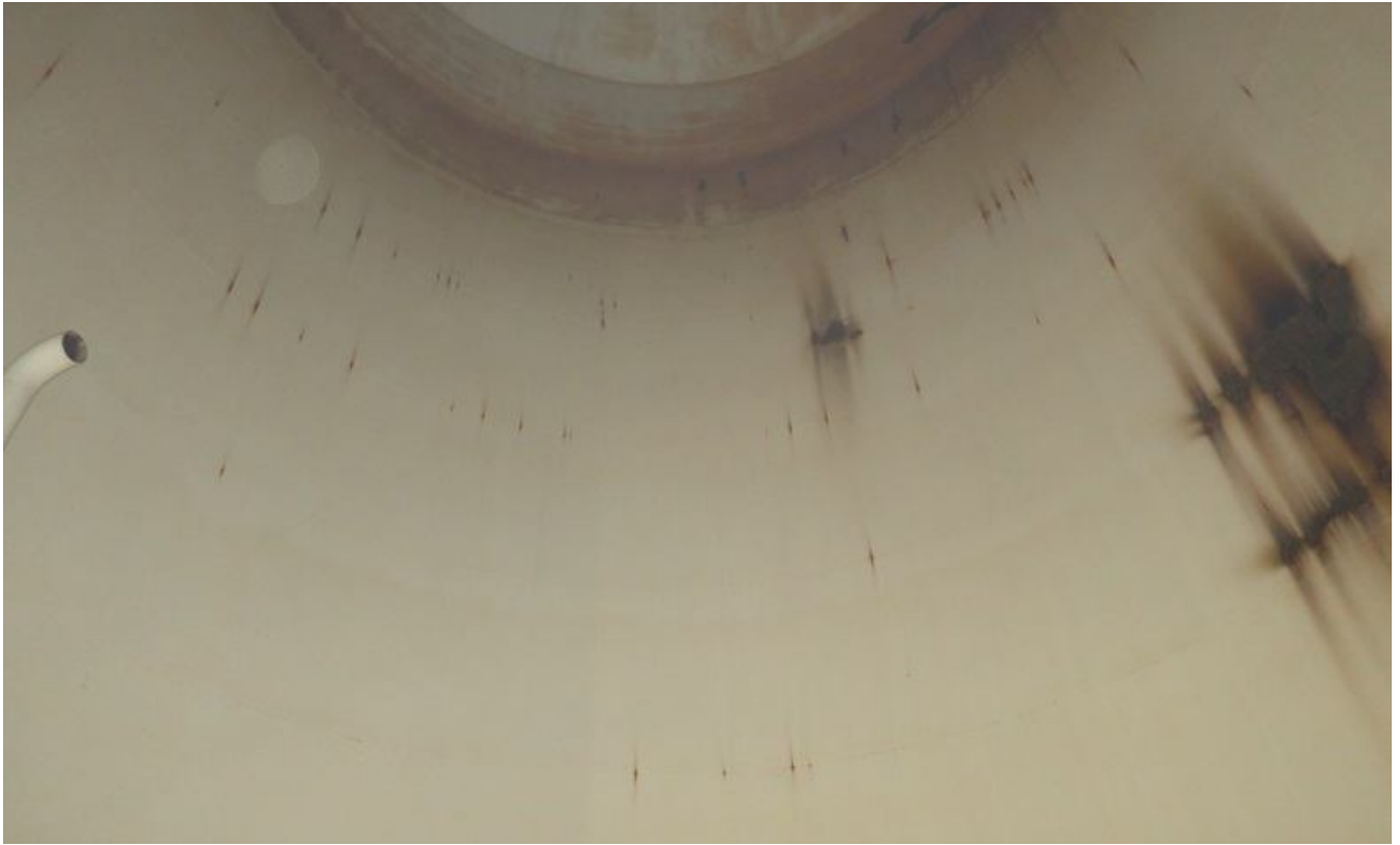
51. Corrosion on interior shell.
