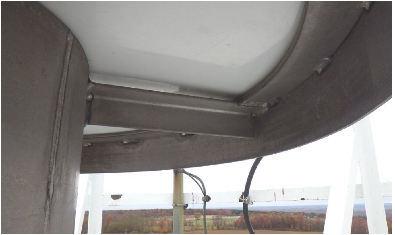
47. Roof vent pallet.
