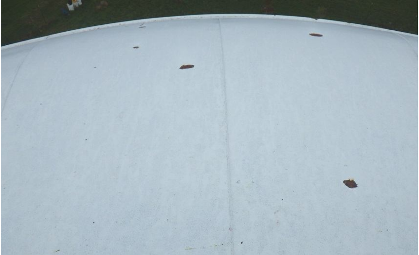
38. Coating failures and rust on exterior roof.
