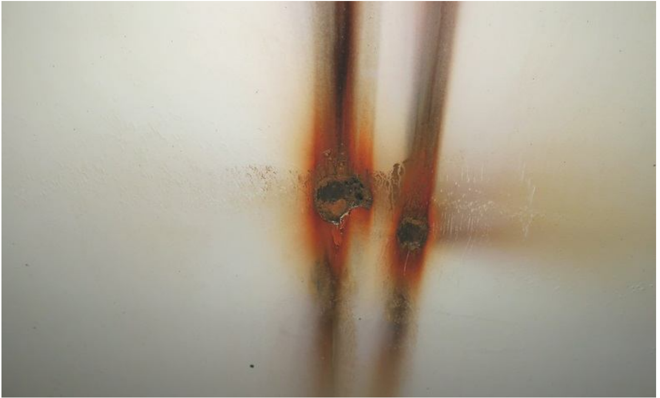
55. Corrosion on interior shell.
