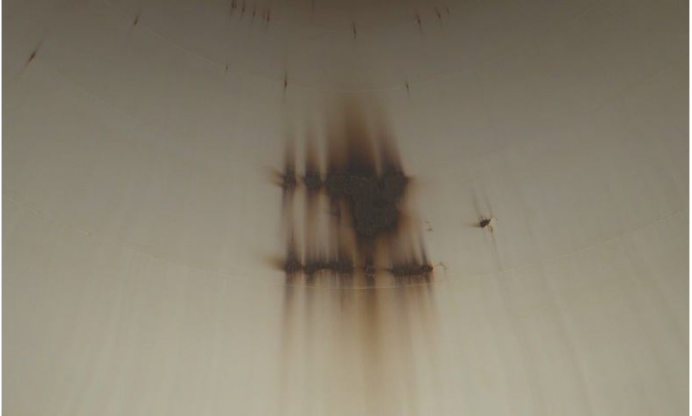
52. Corrosion on interior shell.
