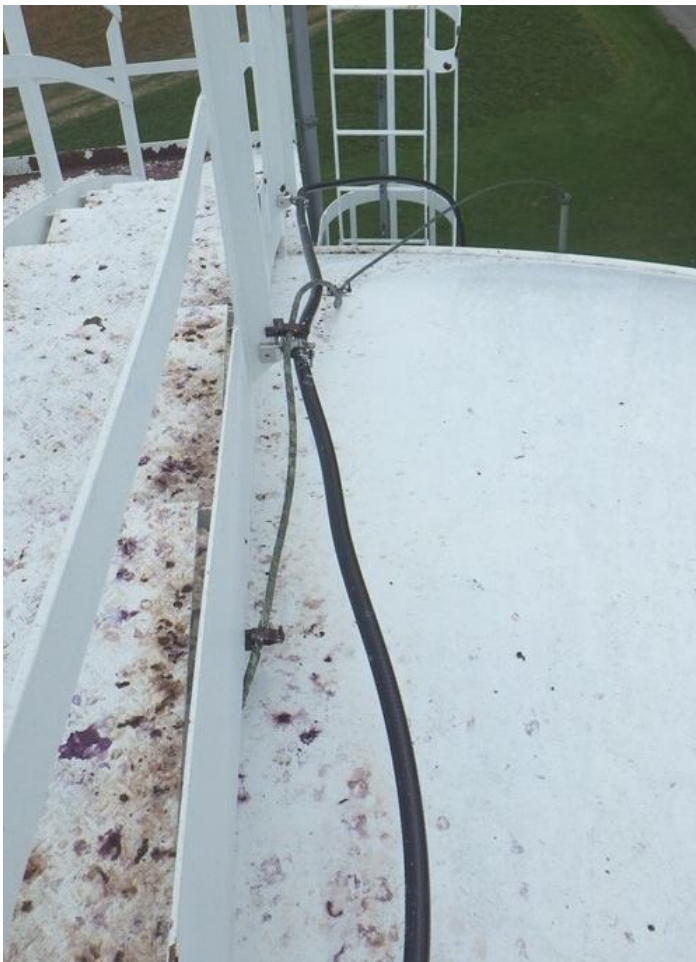
43. Coaxial cable along roof stairs.
