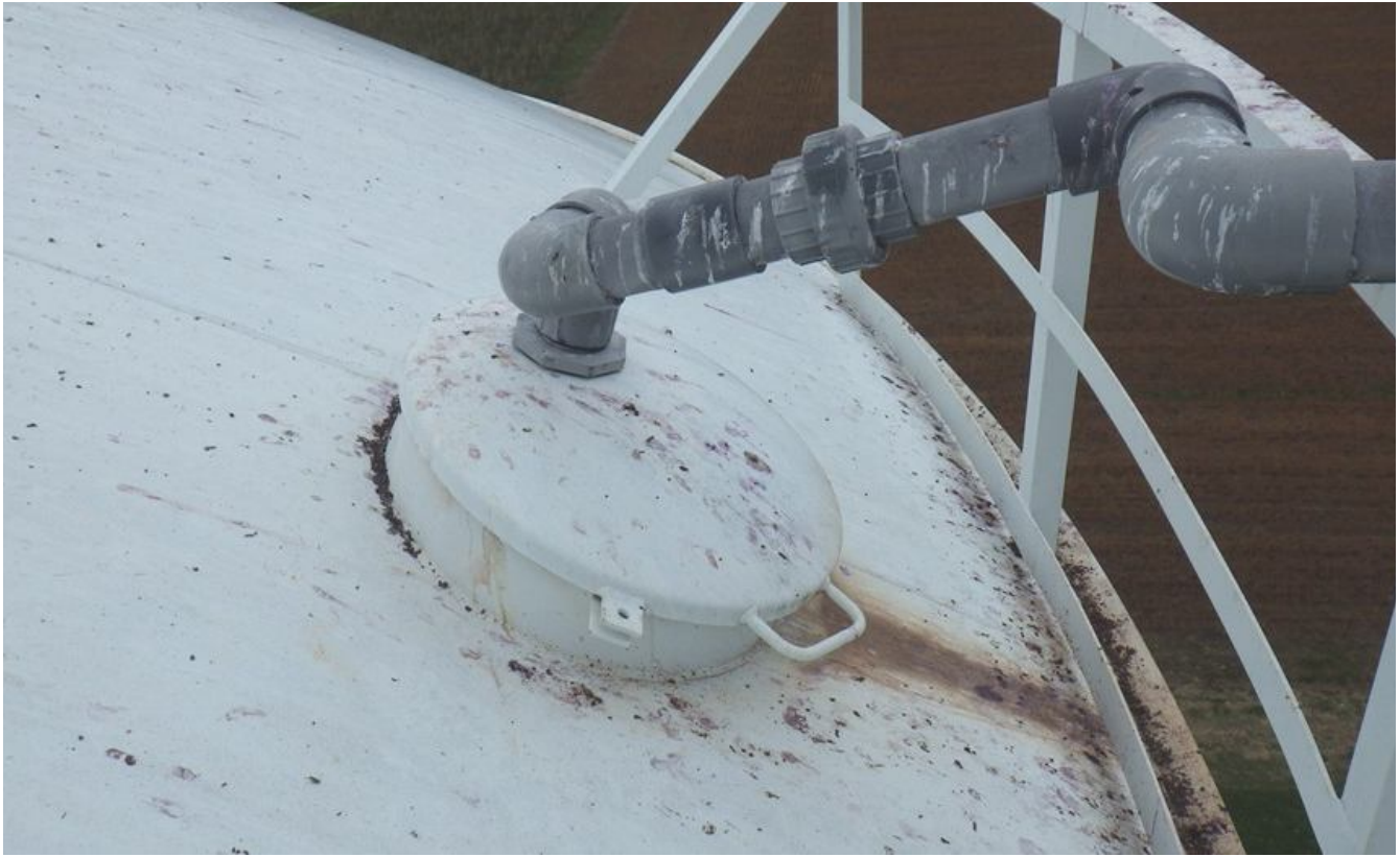
35. Pipe attached to hinged roof manhole cover.
