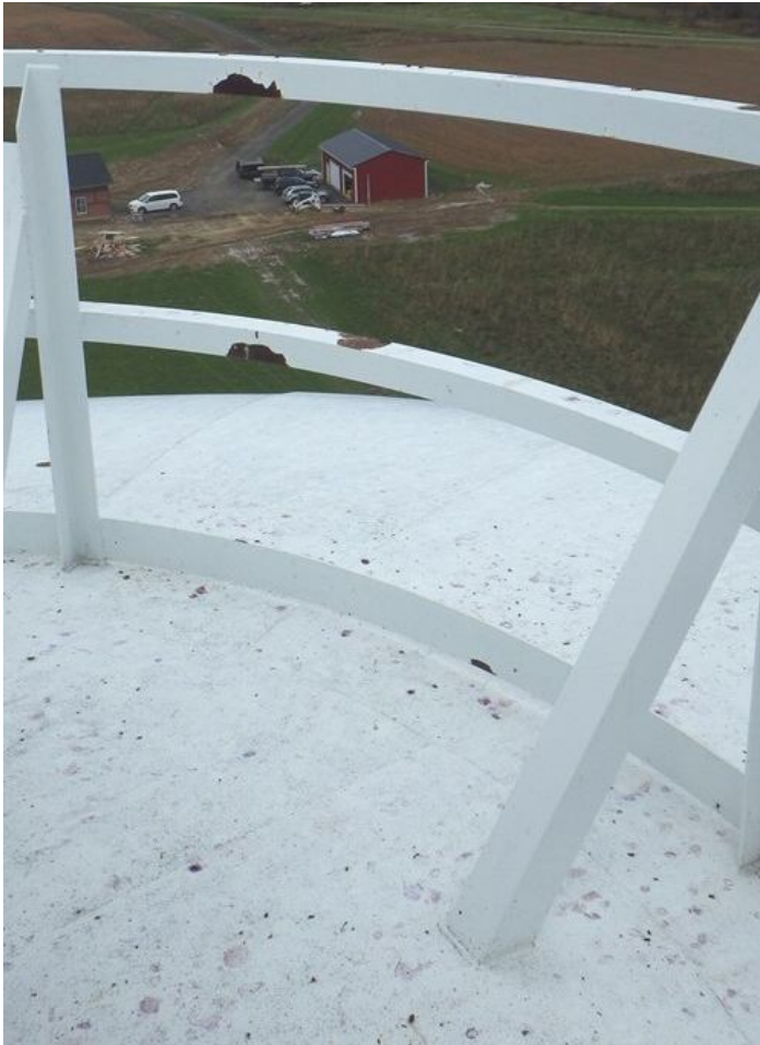
45. Rust on roof safety railing.
