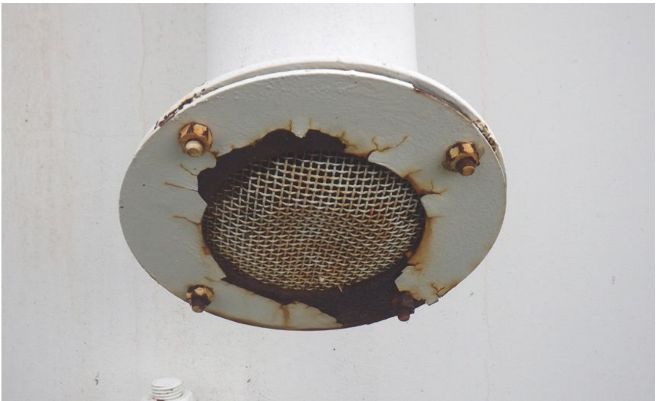
26. Screen at discharge end of overflow pipe. Note rust on flange.
