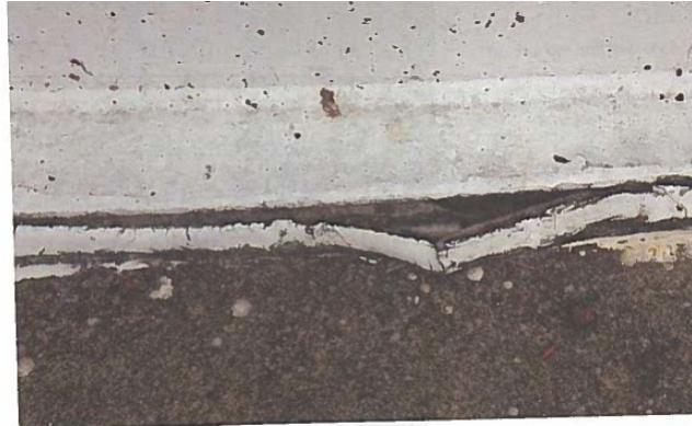
14. Peeled sealant along grout and bottom plate.
