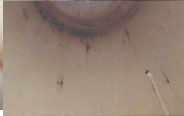
56. Corrosion on interior shell.
