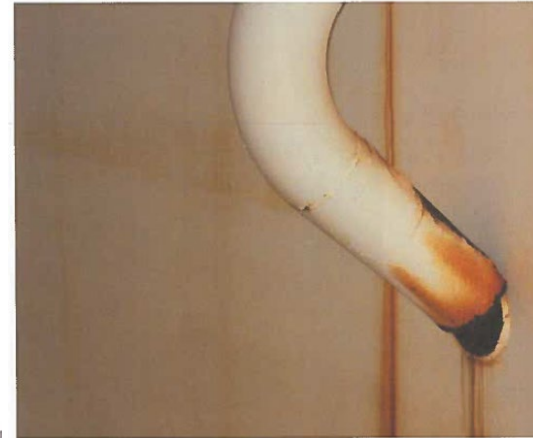
44. Overflow pipe no longer attached to shell.
