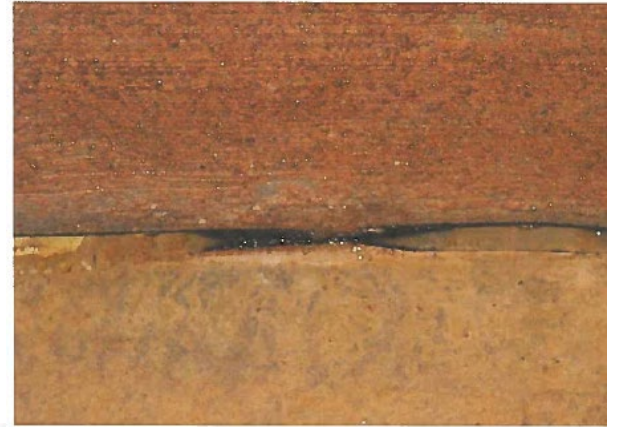
54. Voids in material along shell-to-floor connection.
