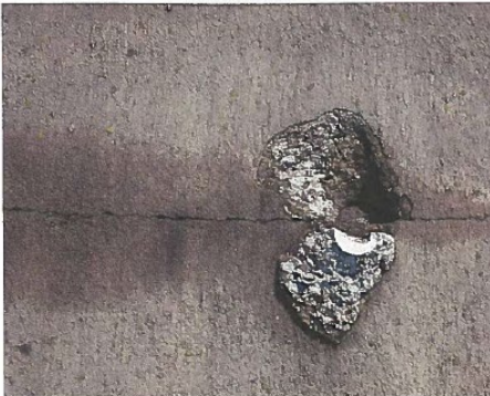
33. Spalling and cracking in roof.
