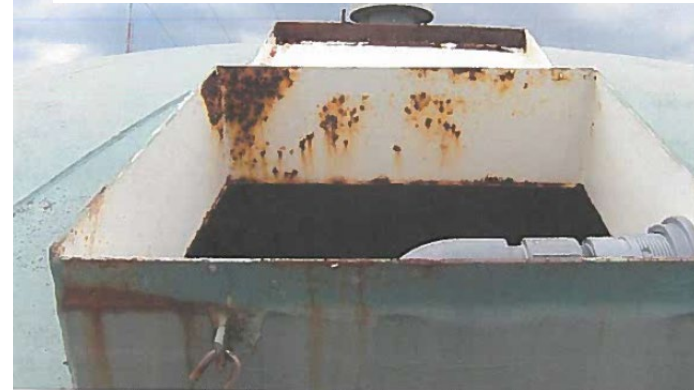
28. Corrosion on roof manhole.
