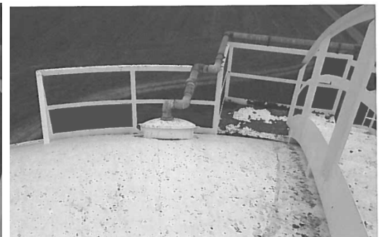
Roof safety railing, platform, stairs, and pipe attached to hinged roof manhole cover.
