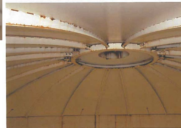
38. Corrosion on roof stiffeners.
