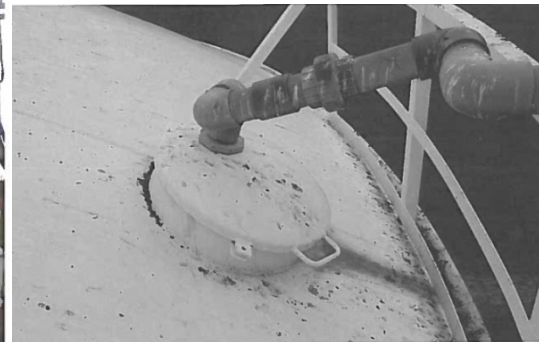
5. Pipe attached to hinged roof manhole cover.
