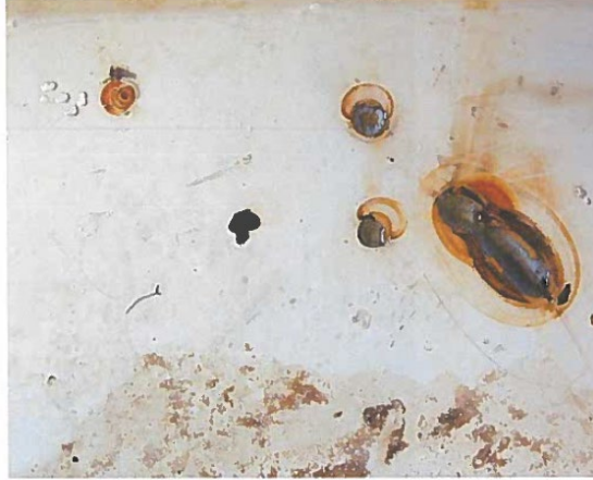
52. Metal loss in floor.
