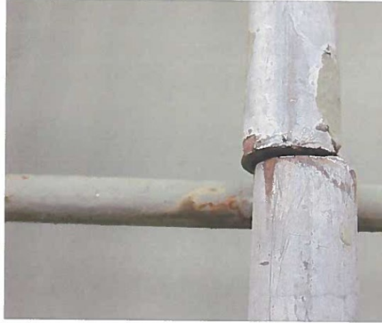
23. Misaligned notched-tubular rail sections.
