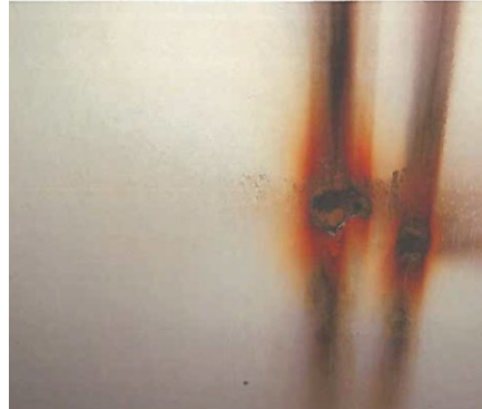
Corrosion on interior shell.
