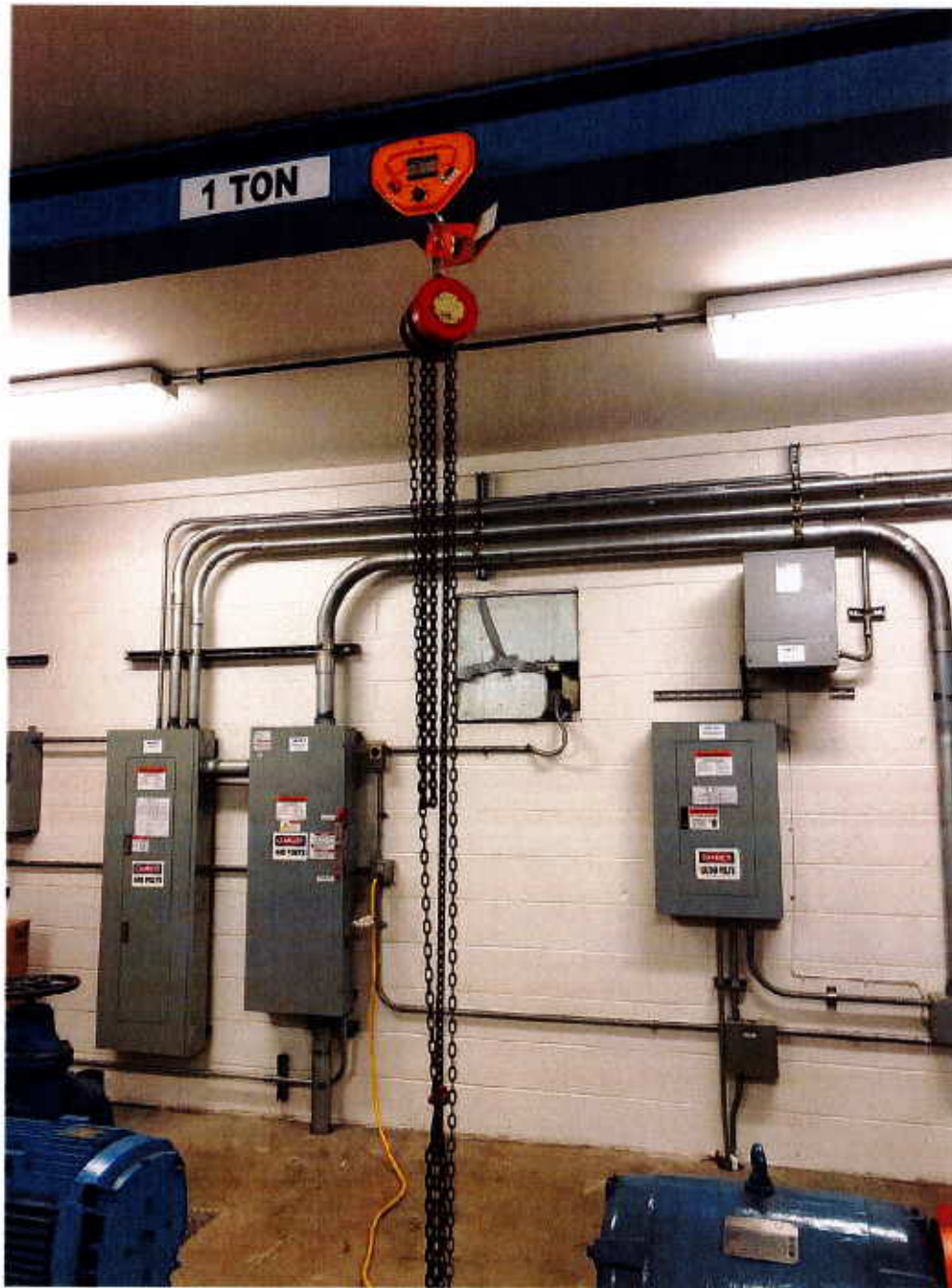
Location: Electrical and Control Panels
