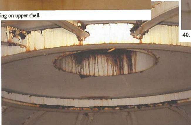
39. Corrosion and metal loss along roof stiffeners and around roof vent opening.
