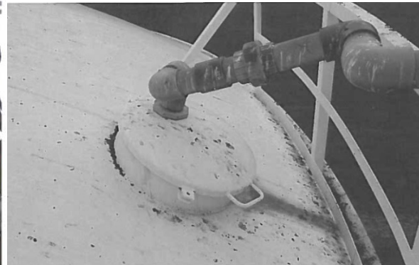
5. Pipe attached to hinged roof manhole cover.
