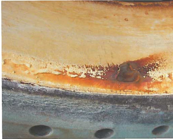
15. Corrosion and metal loss in shell manhole neck.
