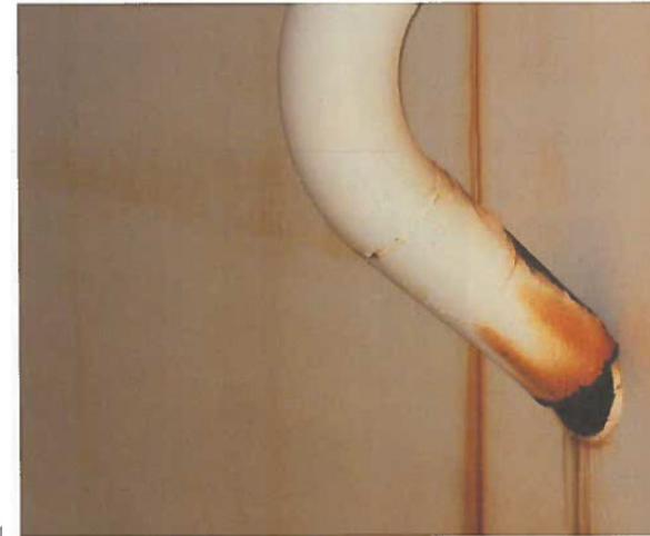
44. Overflow pipe no longer attached to shell.
