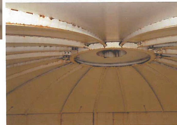
38. Corrosion on roof stiffeners.
