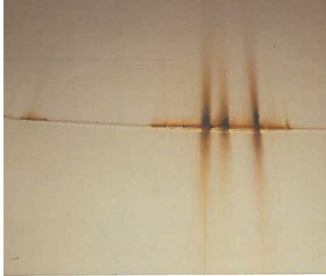
Corrosion along interior shell weld seam.
