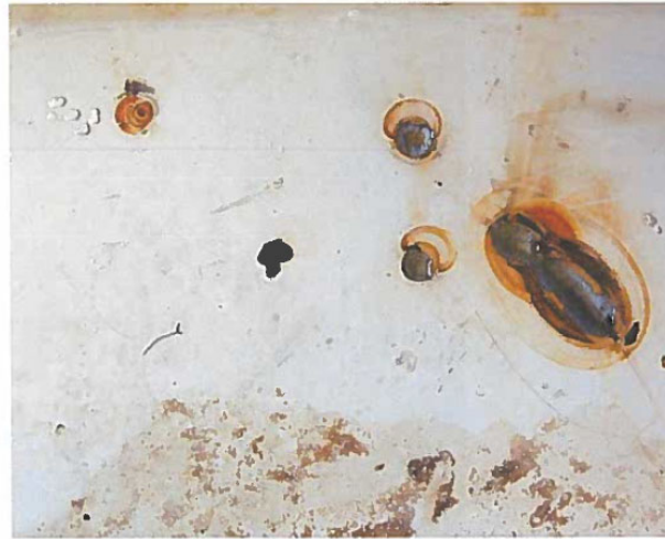
52. Metal loss in floor.
