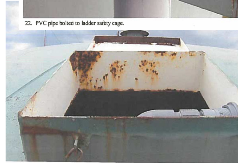
28. Corrosion on roof manhole.
