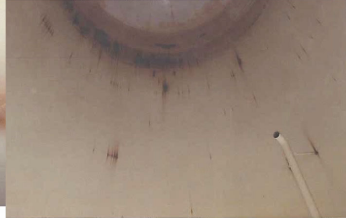
56. Corrosion on interior shell.
