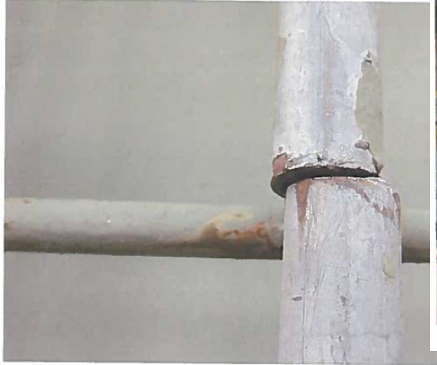
23. Misaligned notched-tubular rail sections.
