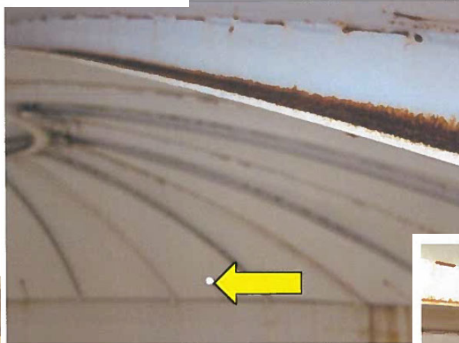
40. Corrosion along roof stiffener. Note daylight at coupling opening.
