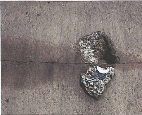
33. Spalling and cracking in roof.
