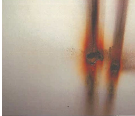
Corrosion on interior shell.
