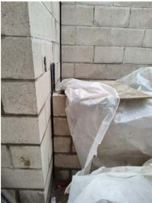
Photo 5: Plumbing chase wall – in progress to be completed when the roof is installed.
