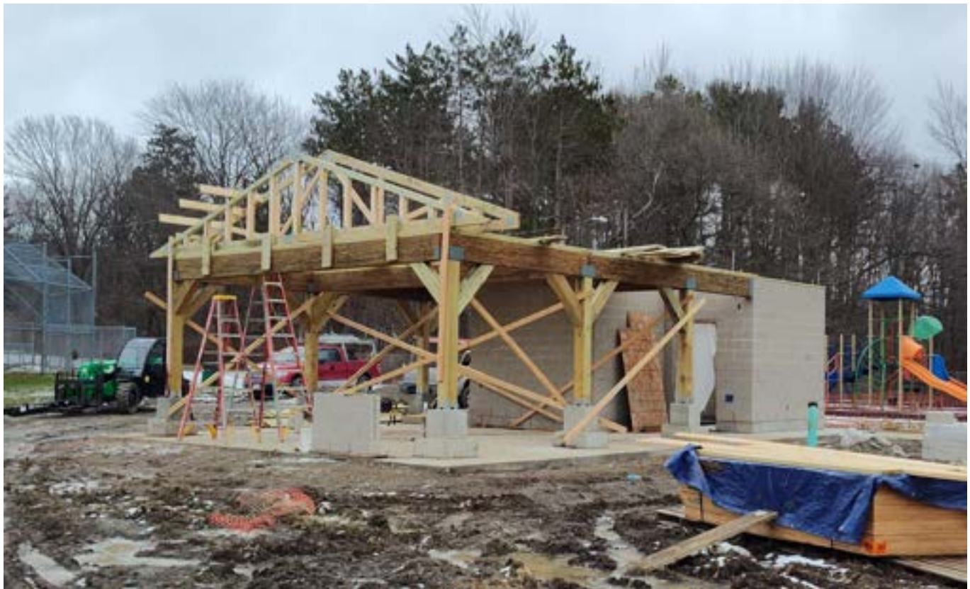
Photo 1: Photo of current site condition. In this photo we see the wood framing in progress. The PSLs are installed and the trusses are in progress.
