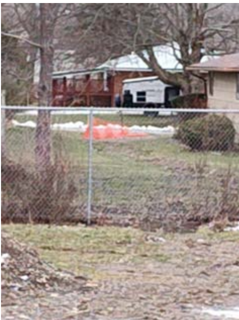
Photo 7: View of neighbors on Parkside still dealing with the orange fence situation in hopes of the RFP & Backflow being installed and their yards restored..
