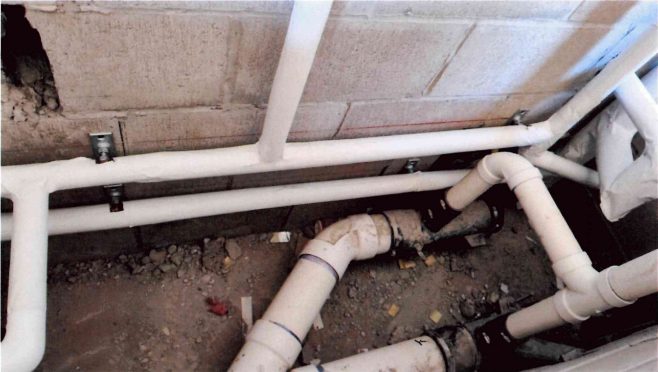
Photo 6: Photo of plumbing pipes in the plumbing chase.
