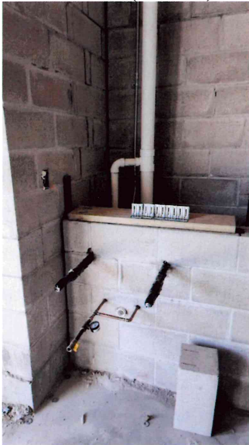
Photo 4: Toilet room progress, air pressure at 76 lbs. in this photo. Once plumbing is reviewed by Tom Murphy the pipes can be insulated and the mason can complete the wall.
