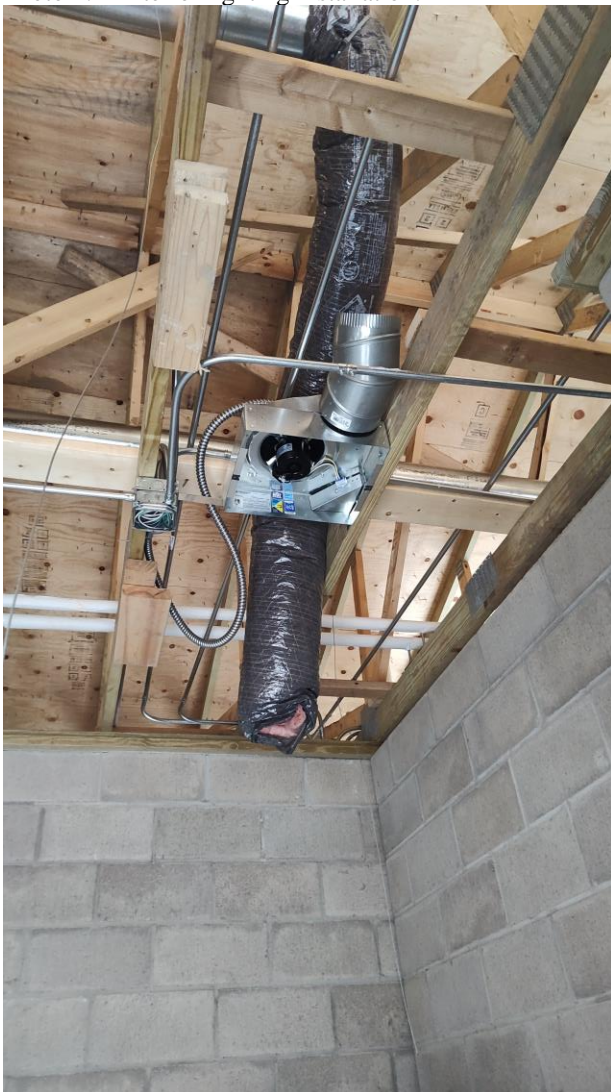
Photo 3: View duct and venting in place for exhaust, also can see the block chase wall complete.
