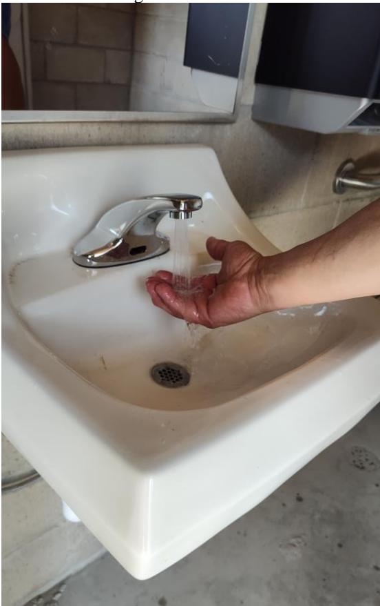
Photo 7: Water was on and working.
