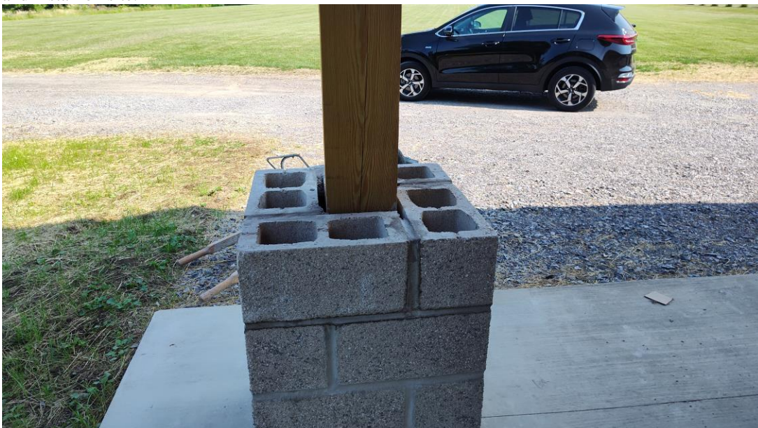
Photo 3: View of precast cap installation in progress- the last pier to receive a cap and be finished.
