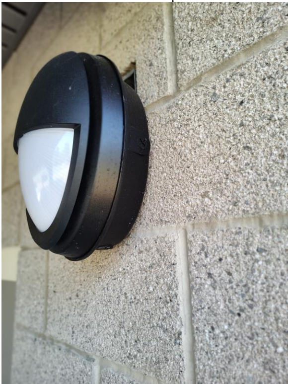
Photo 5: Block that needs to be repaired/ replaced at top of light fixture.
