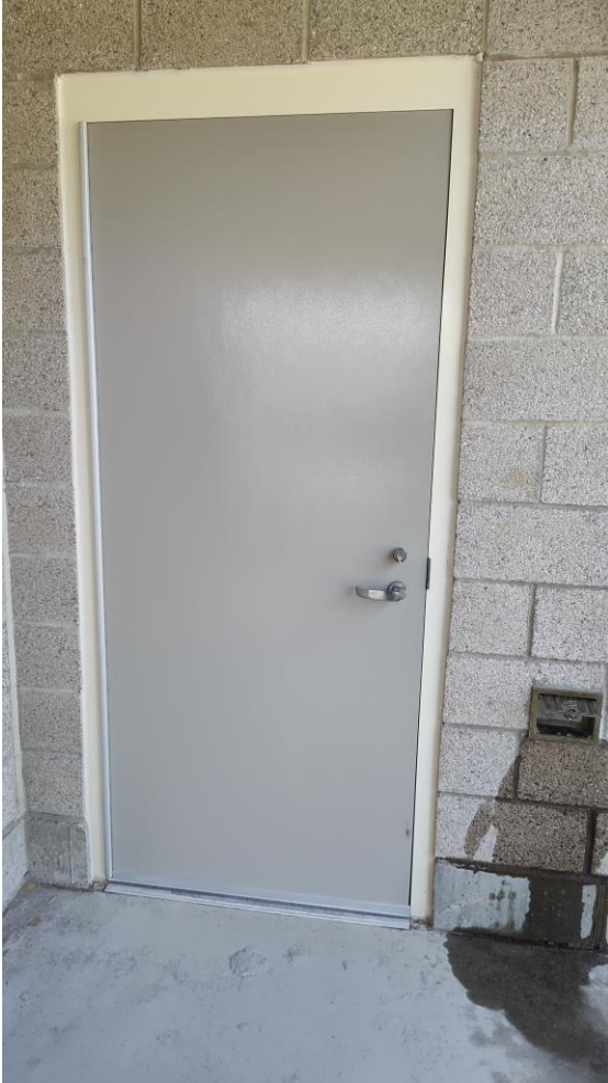
Photo 2: Door & frame installation – Kkogut asked that we do not leave the key sitting there for anyone to take. Shawn Vanderdoes gave Tom Tomaino a secure box with a code to place the key in and install on site.
