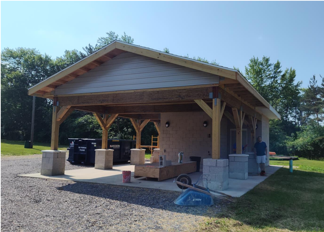
Photo 1: Photo of current site condition. As viewed the cap on the right front pier has not been installed.
