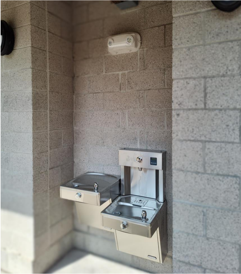
Photo 8: Drinking fountain/bottle filler installation, the bottle filler was not working – contractor to check with plumbing contractor to get it working.
