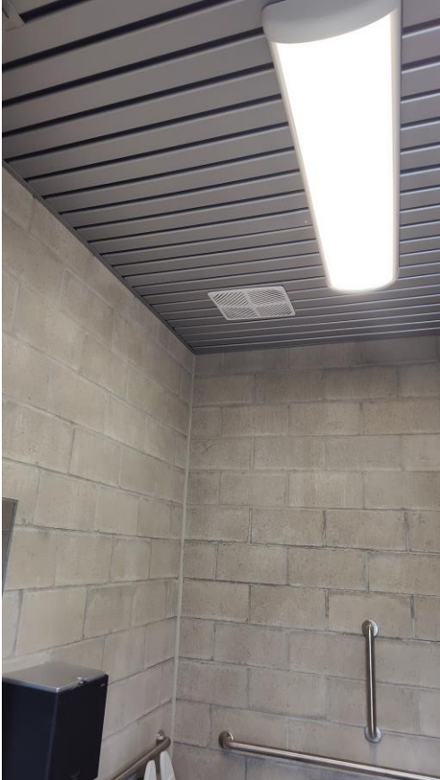
Photo 6: Exhaust fans now in both toilet rooms.
