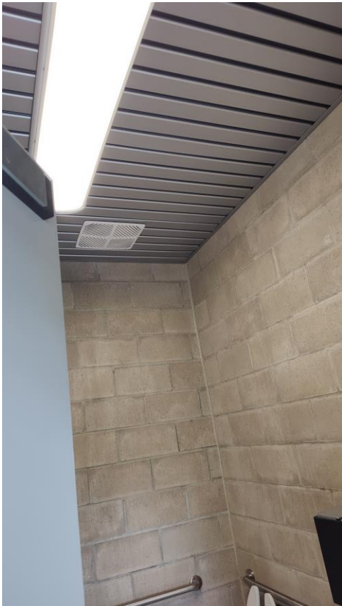
7: Exhaust fans now in both toilet rooms as one was missing during punch list walk-thru.
