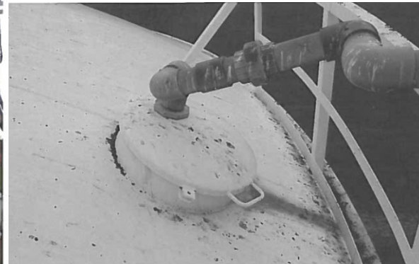
5. Pipe attached to hinged roof manhole cover.
