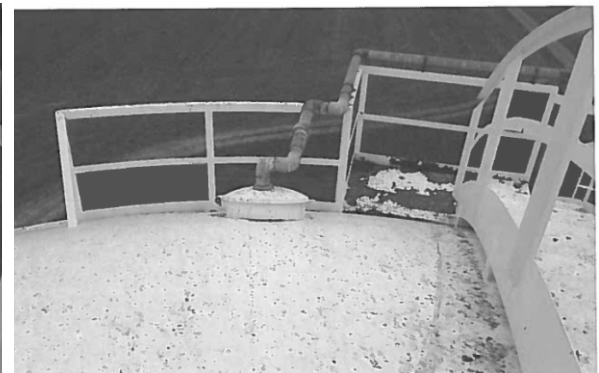
Roof safety railing, platform, stairs, and pipe attached to hinged roof manhole cover.
