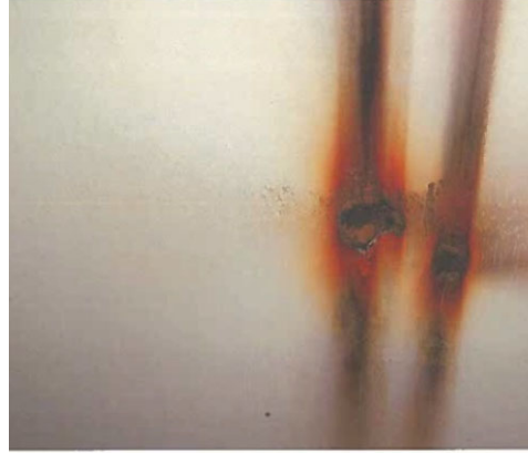
Corrosion on interior shell.
