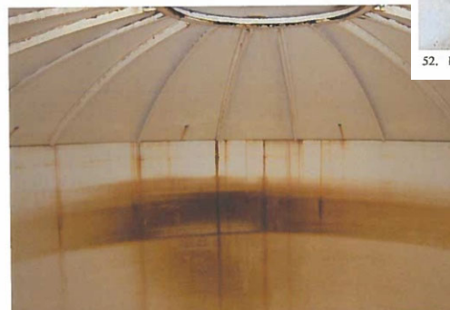
42. Roof and rust staining on upper shell.
