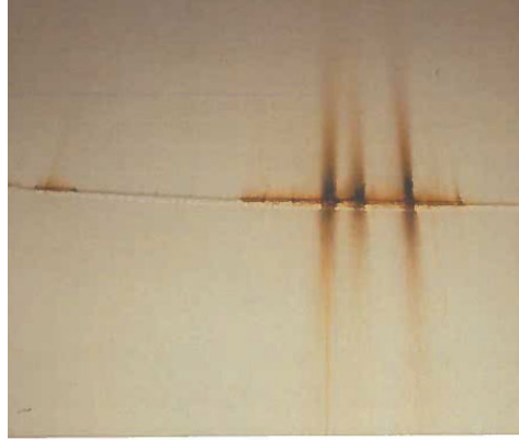
Corrosion along interior shell weld seam.
