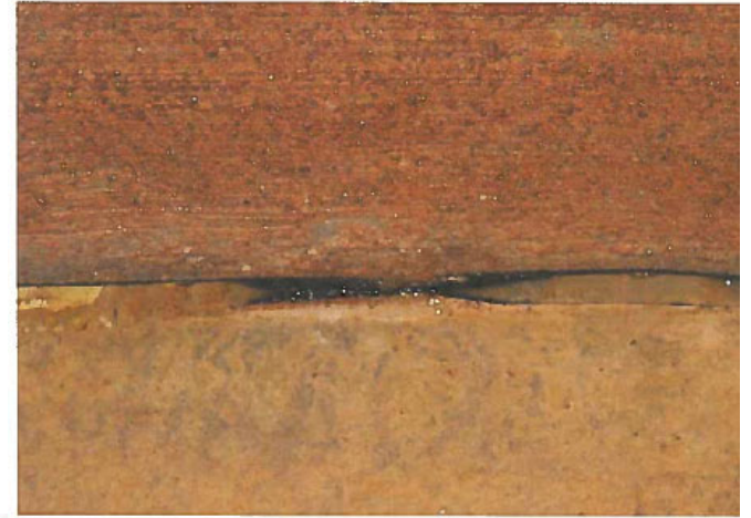
54. Voids in material along shell-to-floor connection.
