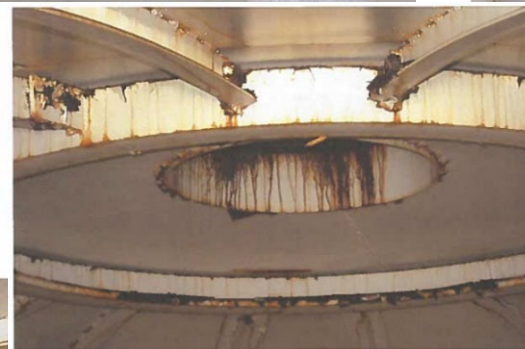
39. Corrosion and metal loss along roof stiffeners and around roof vent opening.
