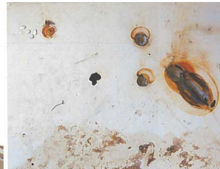
52. Metal loss in floor.
