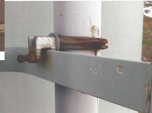
22. PVC pipe bolted to ladder safety cage.
