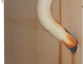
44. Overflow pipe no longer attached to shell.
