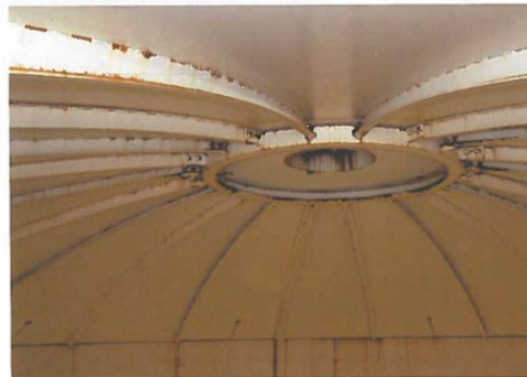
38. Corrosion on roof stiffeners.
