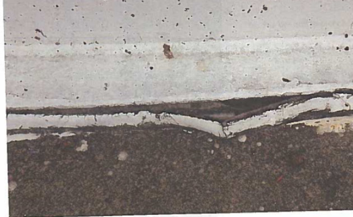
14. Peeled sealant along grout and bottom plate.
