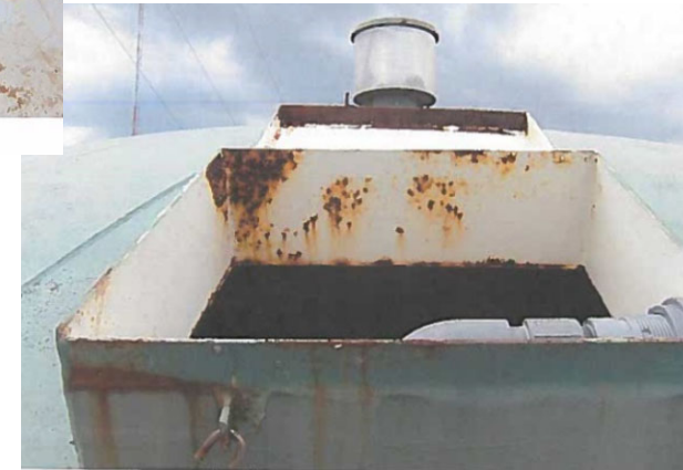
28. Corrosion on roof manhole.
