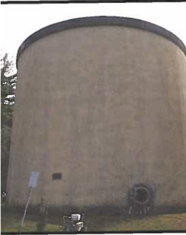
Water District 1 – Crestwood Tank
